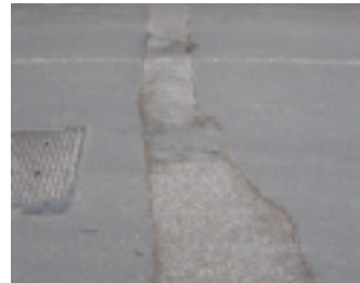
Potholes are a common sight around the Parish
