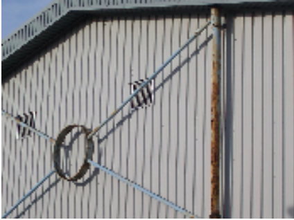
Rusty ironwork on Clarence Road factory.
