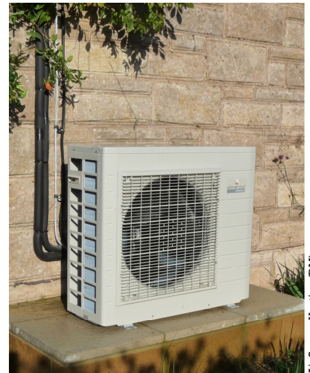
Air Source Heating (DWM)
