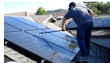
PV panels need to be cleaned at least once per year
