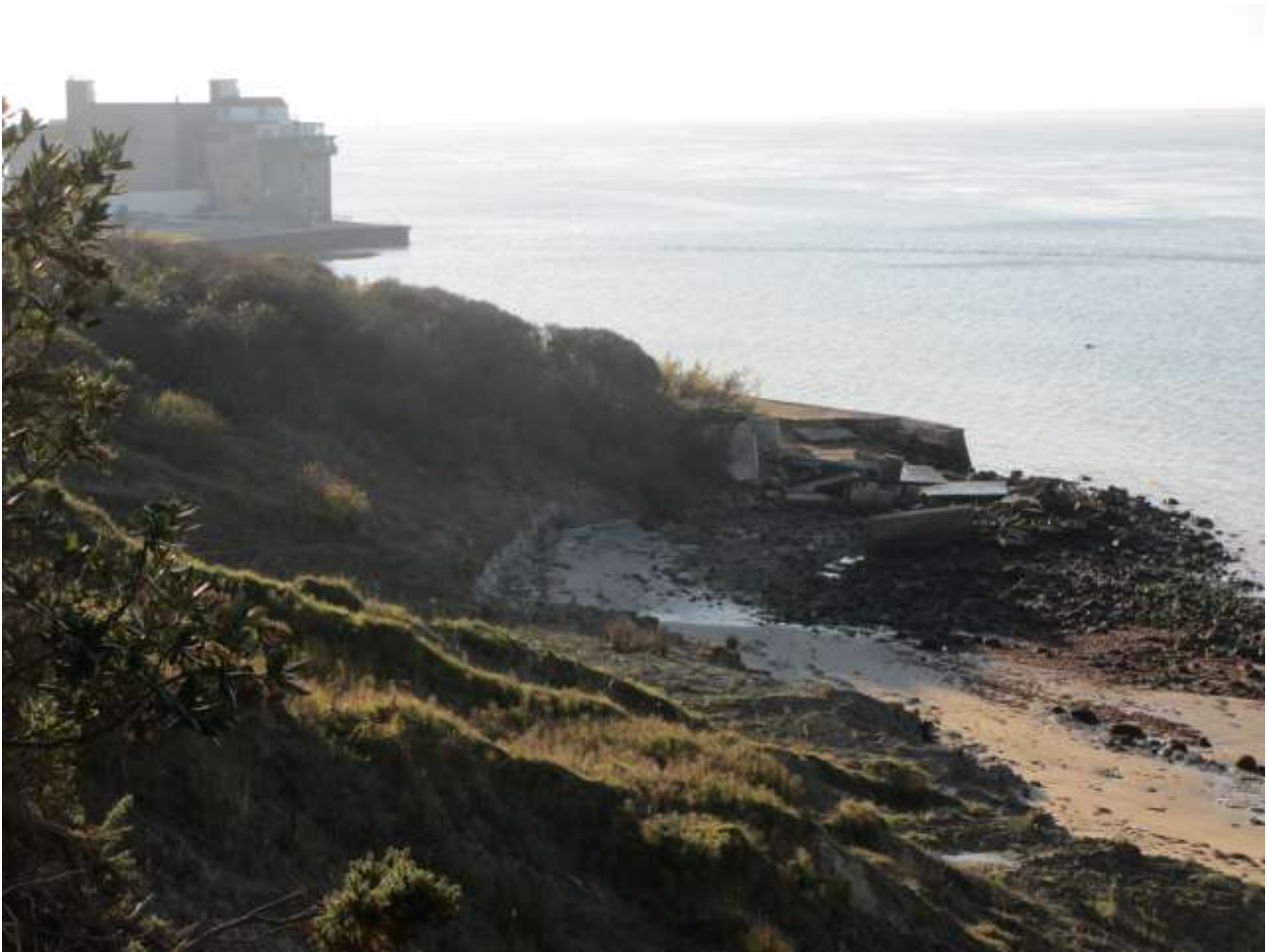
Ageing coastal defences to the north of Fort Albert, at the transition to undefended and eroding coast, 2012
