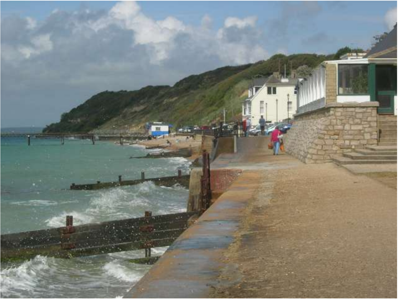
Totland Bay, where waves attack the seawalls and cliff reactivations have slumped over the seawalls. Photo taken in July 2009, showing the cliff-line in the distance prior to the December 2012 landslide (discussed below).
