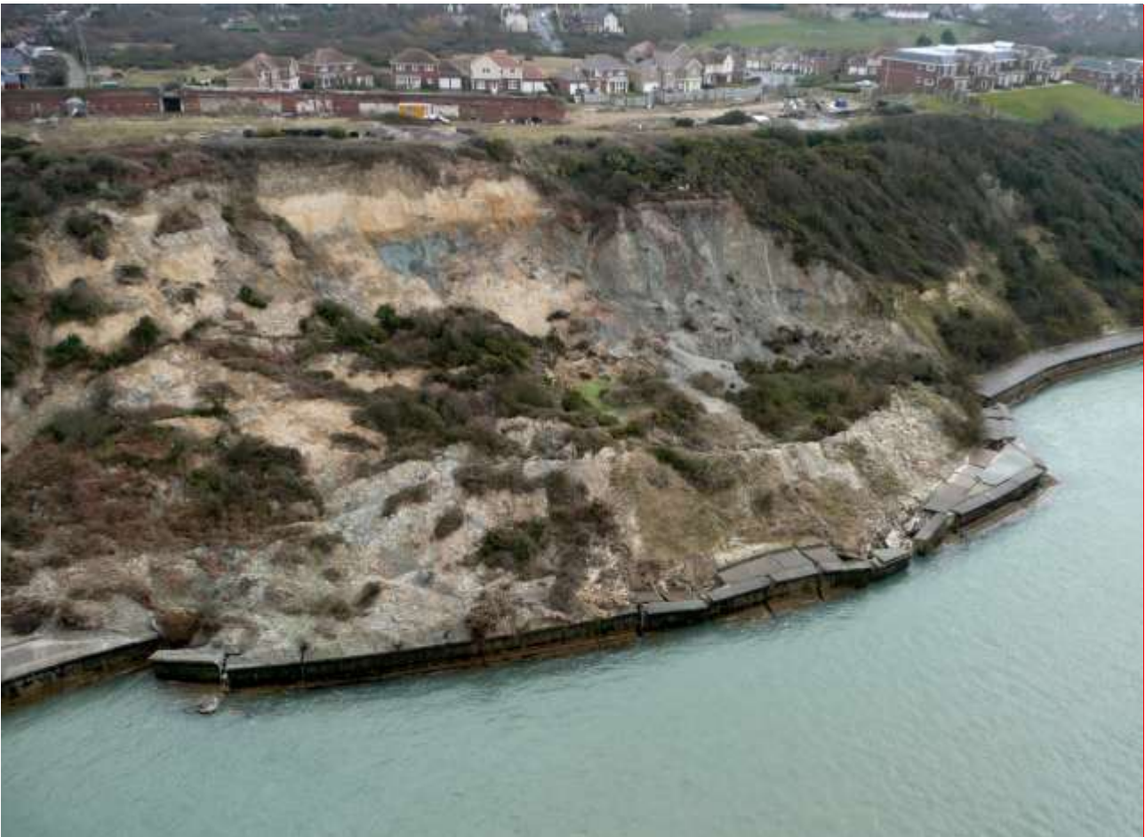
Aerial photograph of the Totland landslide, which is over 100m in length, taken in April 2013 (i.e. three months after the slide began). The landslide has continued moving since then. (Photo courtesy of HM Solent Coastguard).
