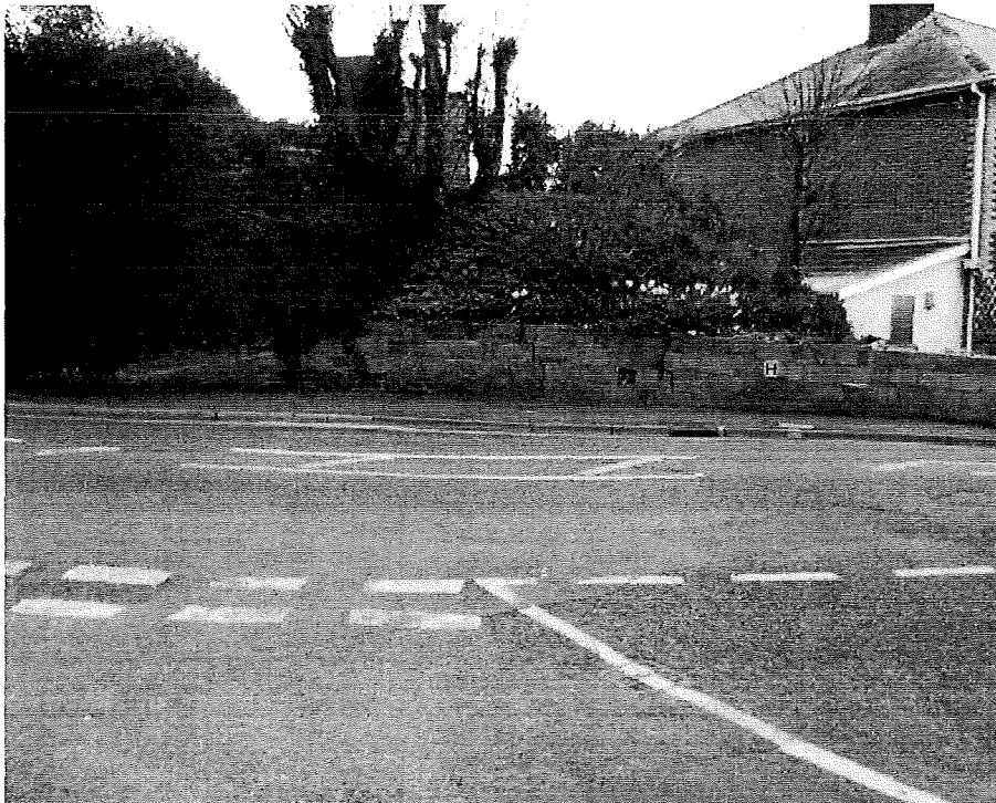
Figure 4b, Movement and cracking of wall at south side of graben opposite Upper Gills Cliff Road
