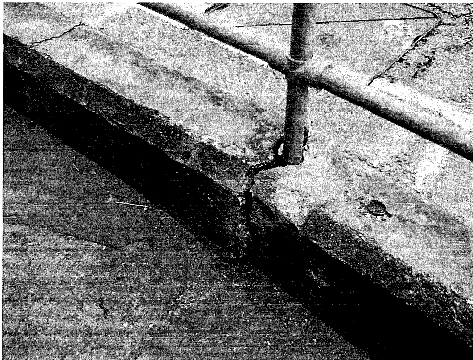
Figure 4d, Cracking of rigid handrail base, north side of graben
