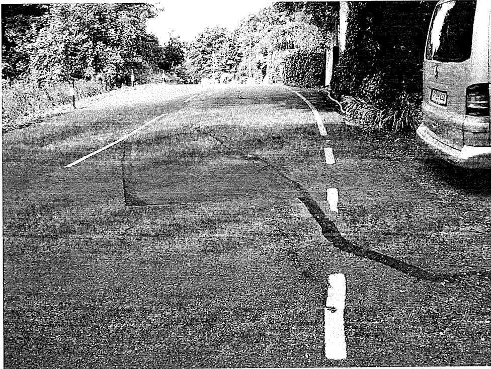
Plate 5: Cracking along lateral shear, Woodlands Area 4
