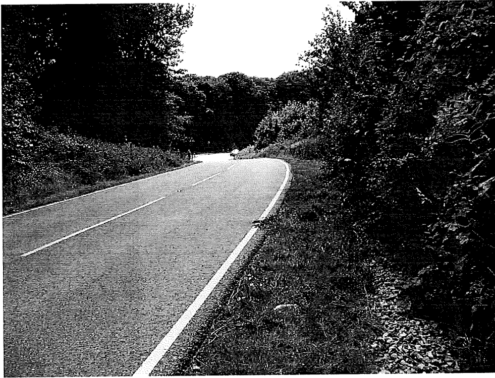
Plate 1: Road condition, Area 1 Beauchamp
