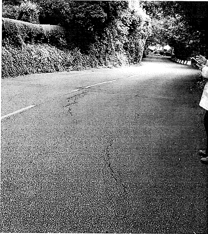
Plate 7: Localised cracking in westbound carriageway, Area 5 St Lawrence West
