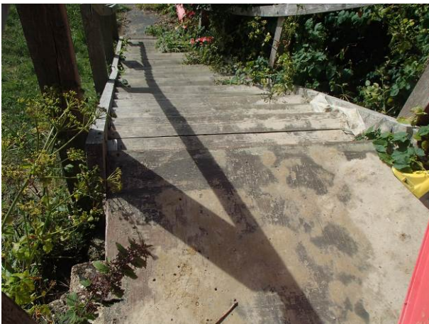
Displacement of timber steps
