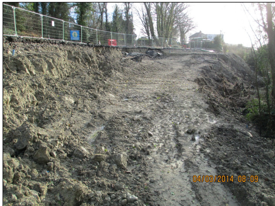
Figure 1b. Site 10 Caravan Park Geological Failure: Failure cutting across the footprint of the westbound carriageway and along existing cracks.
