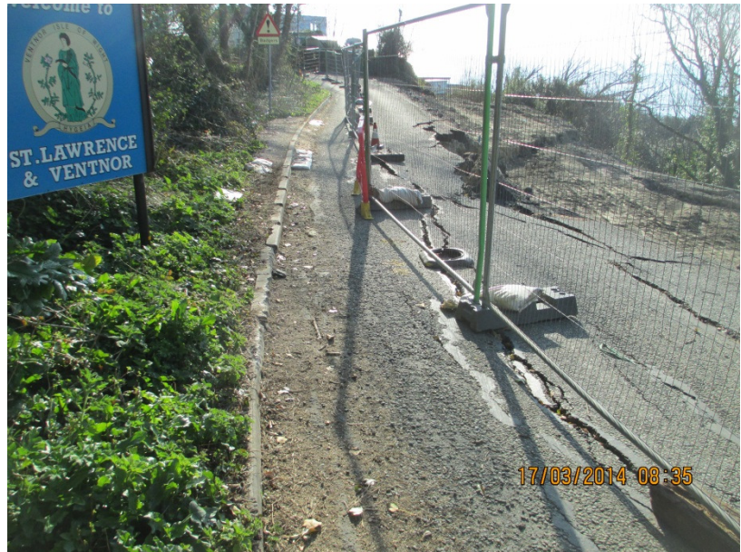
Figure 2b. Site 10 Caravan Park Geological Failure: Barriers through the centre of the site.
