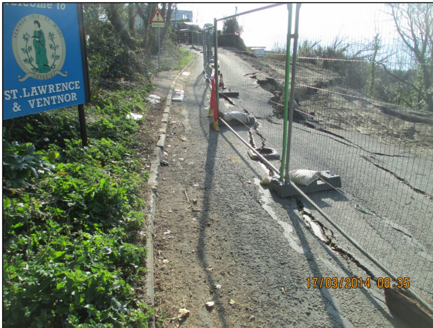
Figure 1a. Site 10 Caravan Park Geological Failure: Failure of the carriageway on the eastbound side and retrogression inland.
