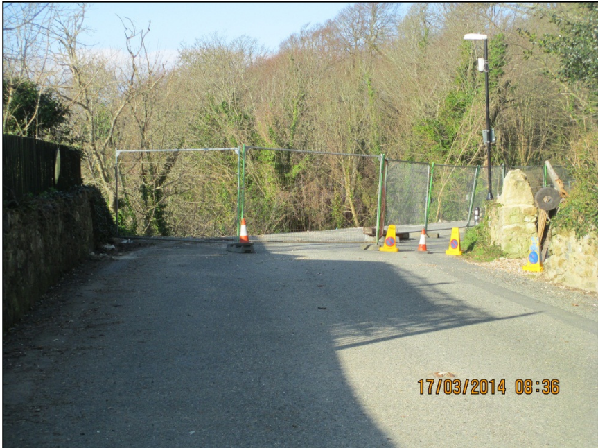
Figure 2c. Site 10 Caravan Park Geological Failure: Barriers at the eastern extent of the site.
