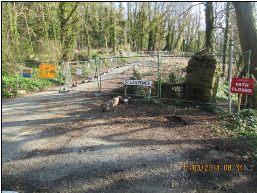
Figure 2a. Site 10 Caravan Park Geological Failure: Barriers at the western extent of the site.
