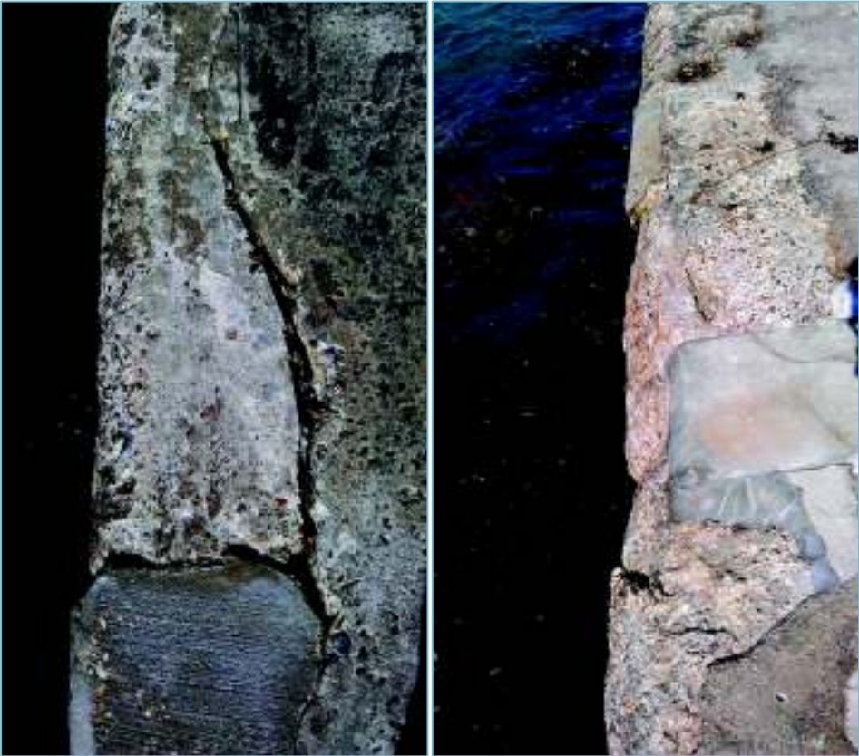
Figure 8.1: Defence Section 1 - Cracks along seawall crest.
