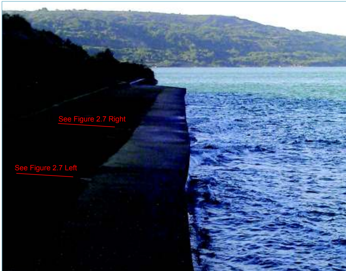
Figure 8.6: Defence Section 3 – Potential seawall movement
