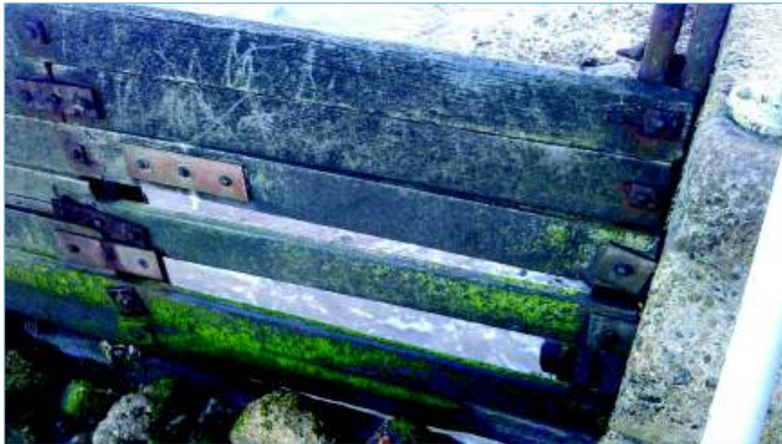
Figure 8.13: Defence Section 4 – Missing planks at inshore end of 2 nd groyne.
