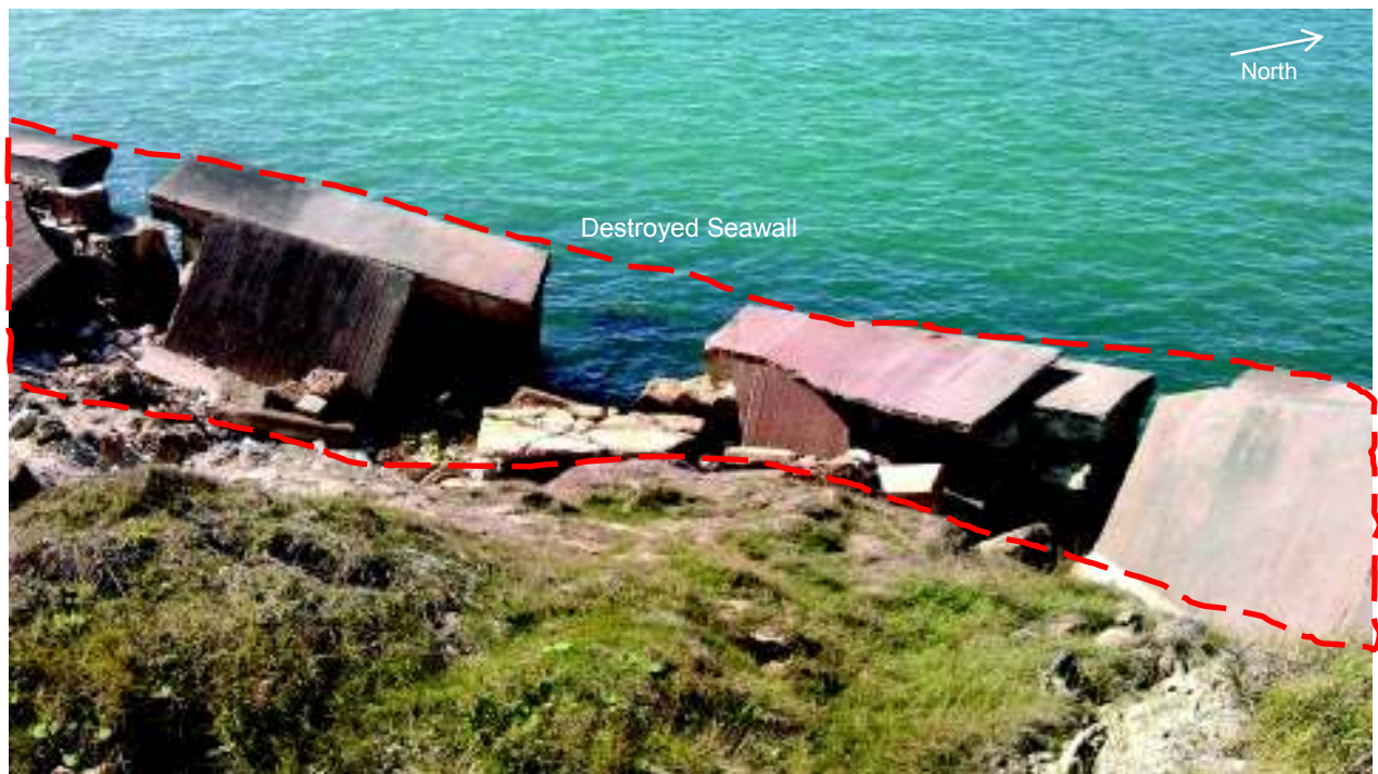
Figure 3.3: A section of the seawall fronting the landslide in September 2013 when the defence condition survey was carried out.
