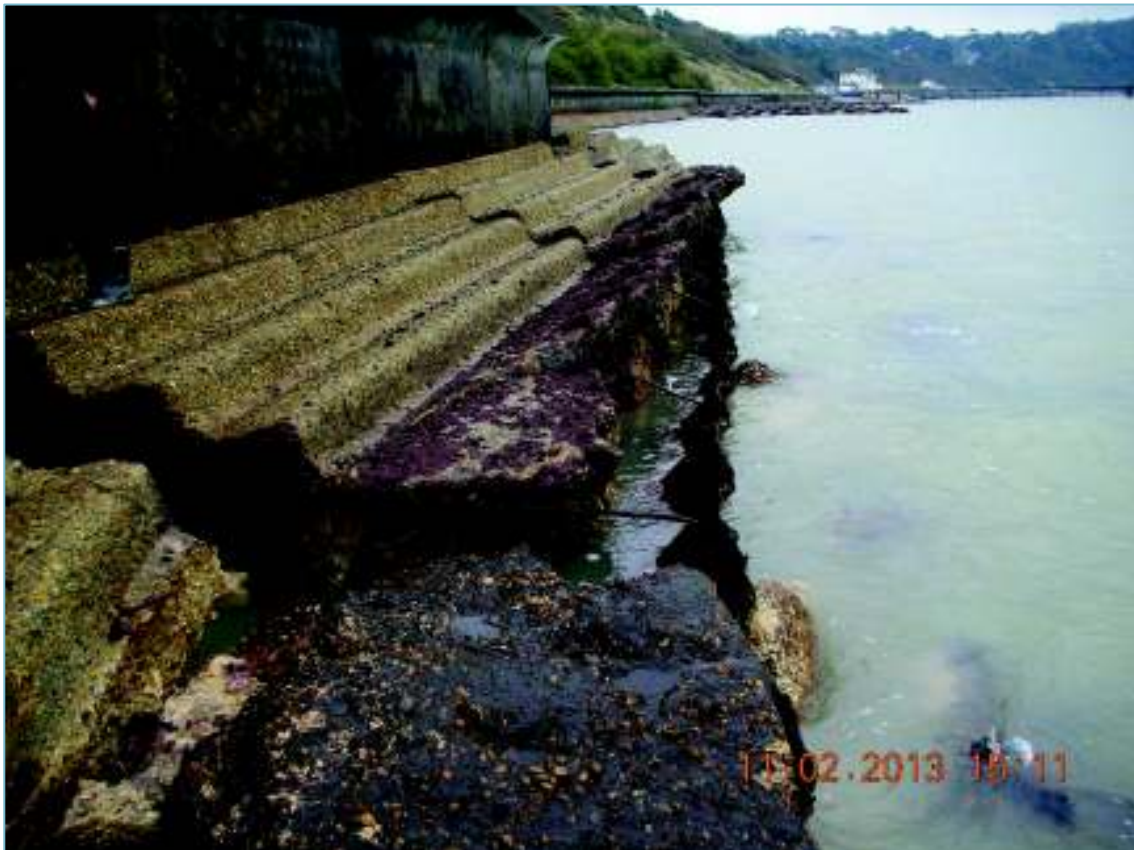
Figure 8.17: Failed seawall central section at low water – view looking towards Totland Bay (11 th February 2013)
