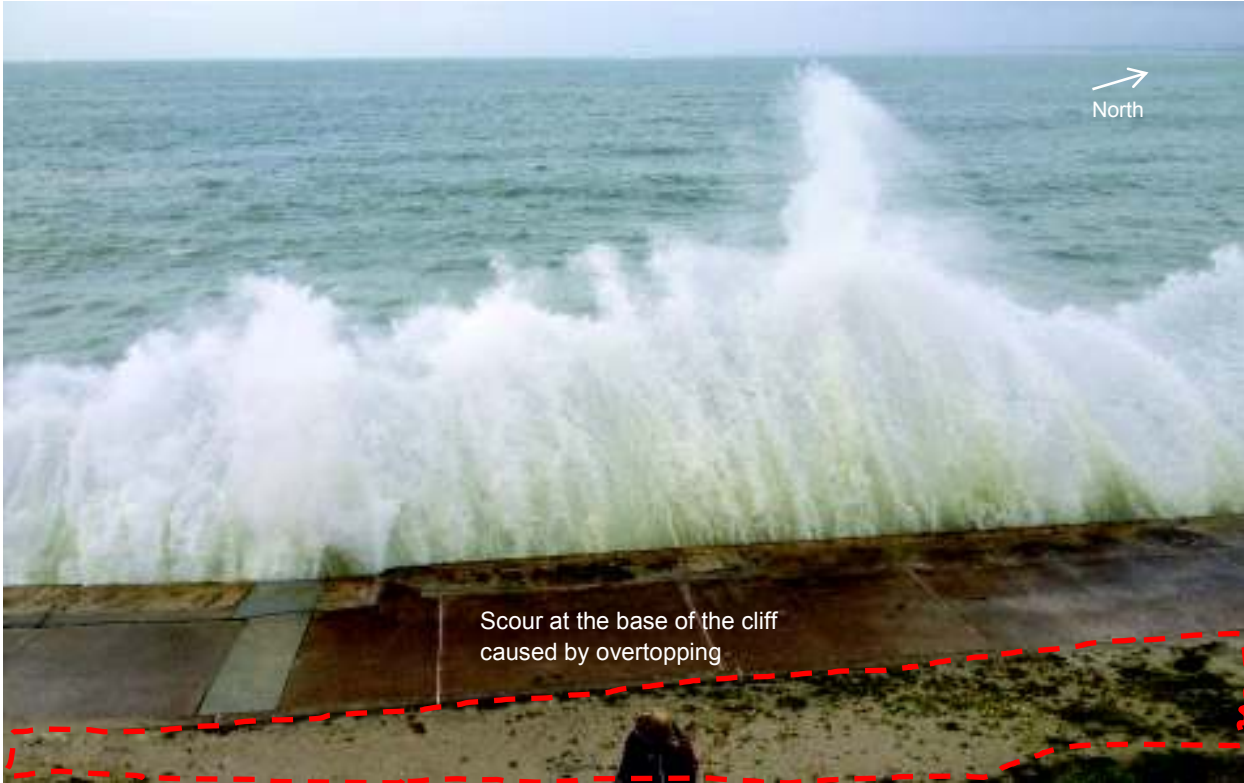
Figure 3.4: Overtopping of the seawall and scour caused at the base of the cliff.
