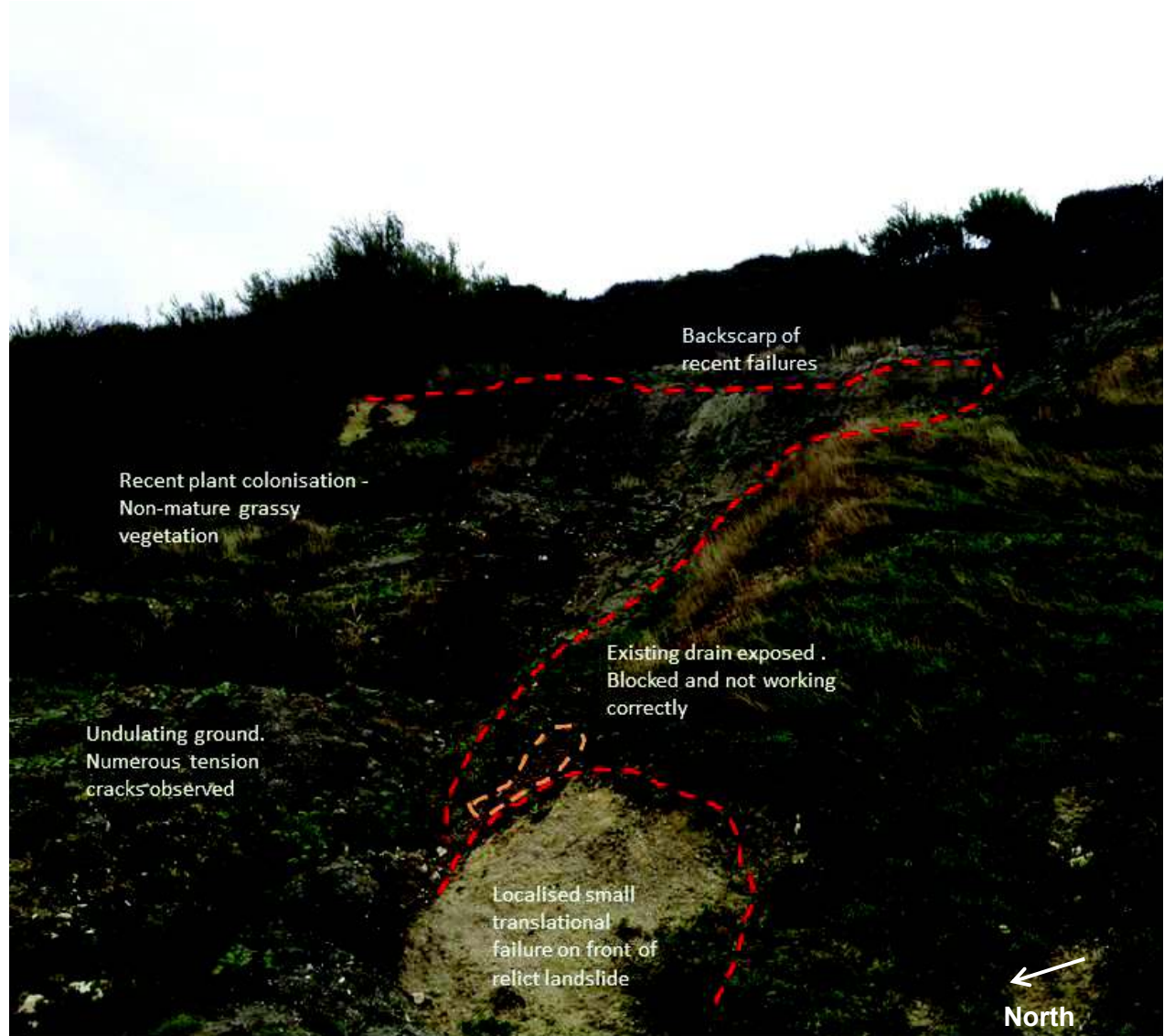
Figure 4.6: The recent surficial instabilities within the section of frontage to the south of the landslide.
