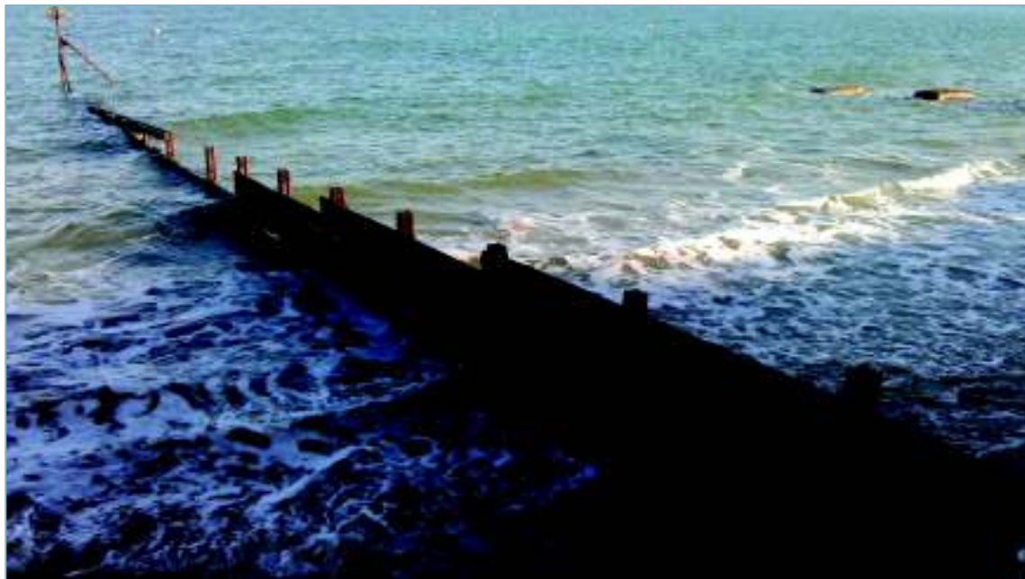
Figure 8.12: Defence Section 4 - Timber groyne with missing planks towards offshore end.
