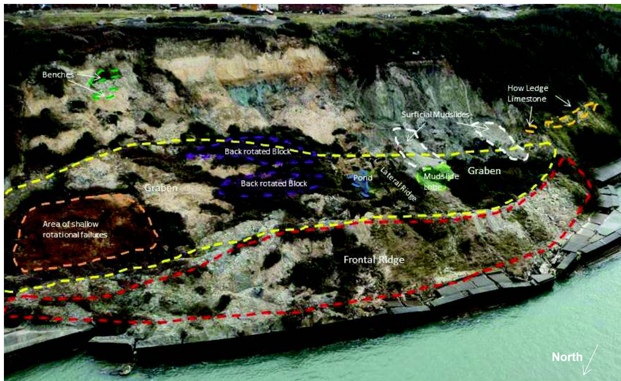
Figure 4.3: Some of the main features observed on the landslide. Image from the cliff top looking down over the landslide
