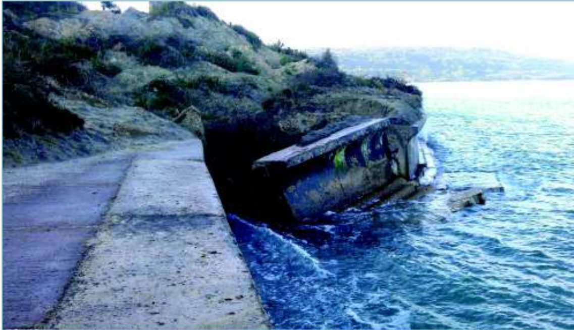
Figure 8.5: Defence Section 3 – Seawall adjacent landslide
