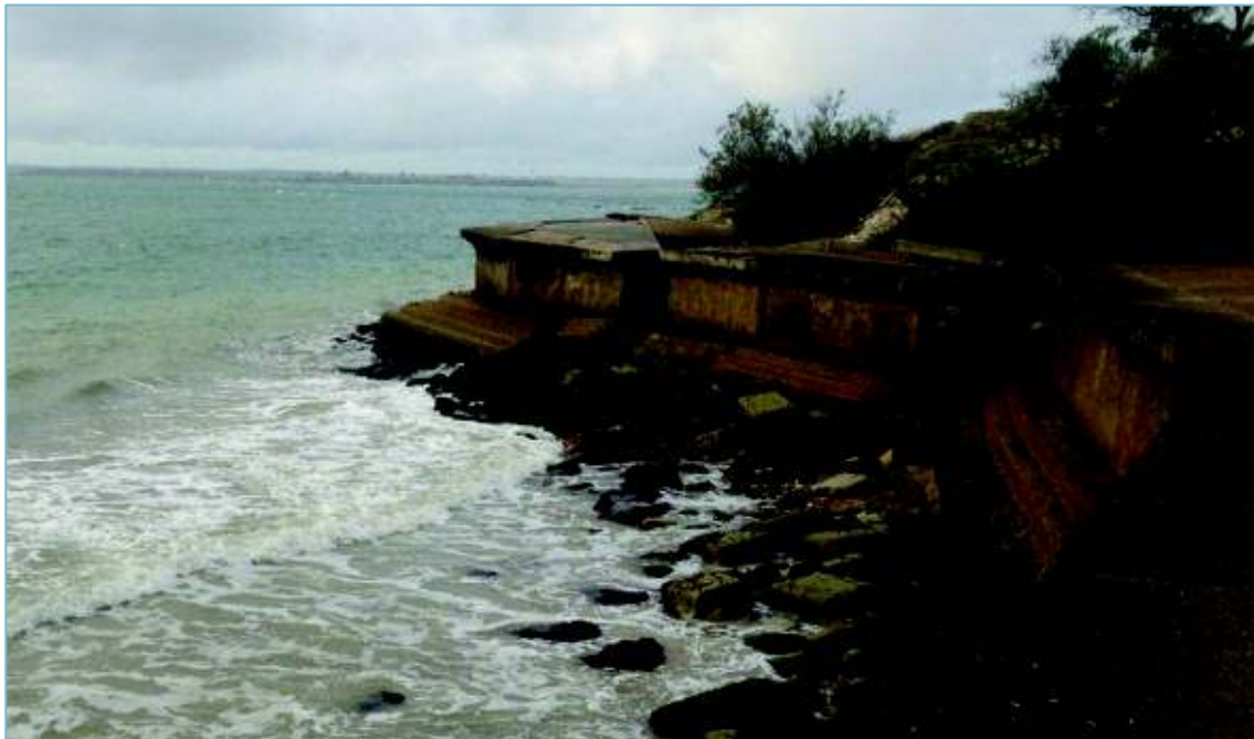
Figure 8.16: Failed seawall – viewed from Totland Bay looking north (19 th September 2013).
