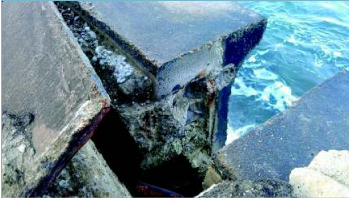
Figure 8.15: Cross section of failed seawall (20 th September 2013)
