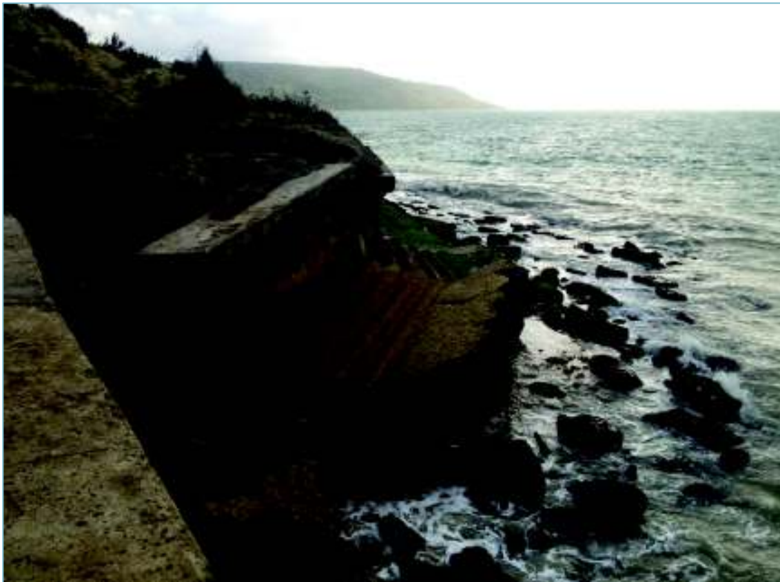
Figure 8.18: Failed seawall – viewed from Colwell Bay extent of landslide looking south (19 th September 2013)
