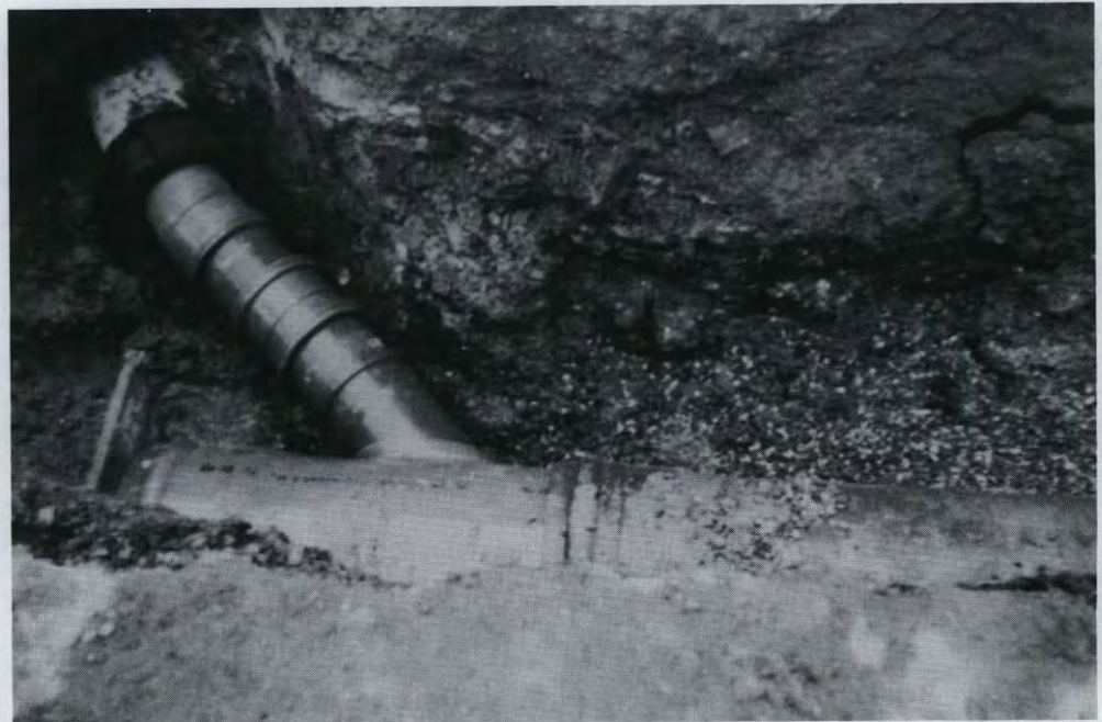
Plate 17. Flexible joint connections to main sewer.
