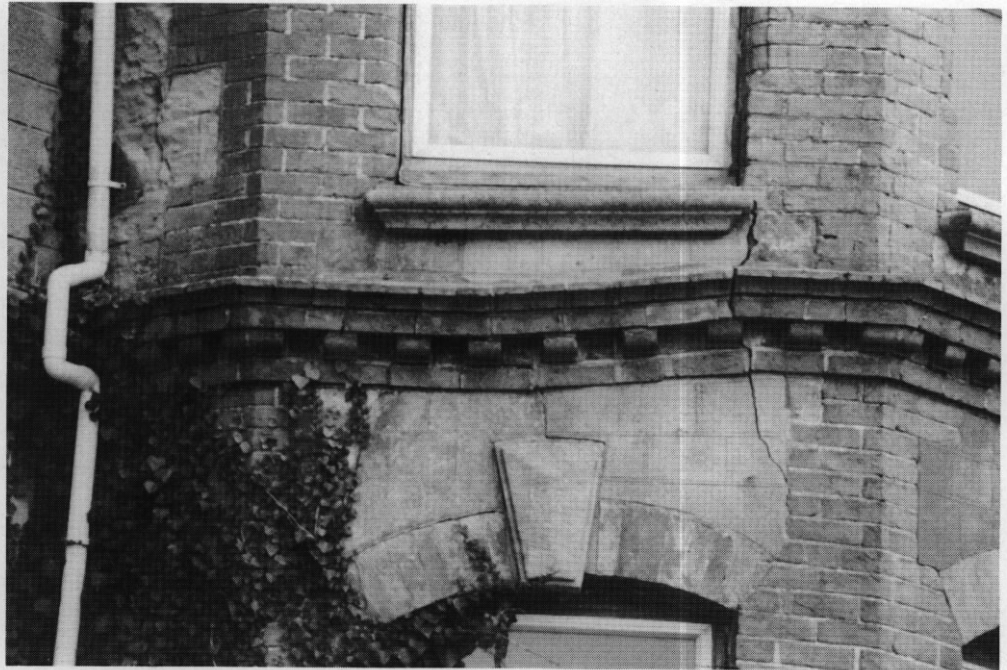
Plate 9. Structural damage to string course, arch and keystone.
