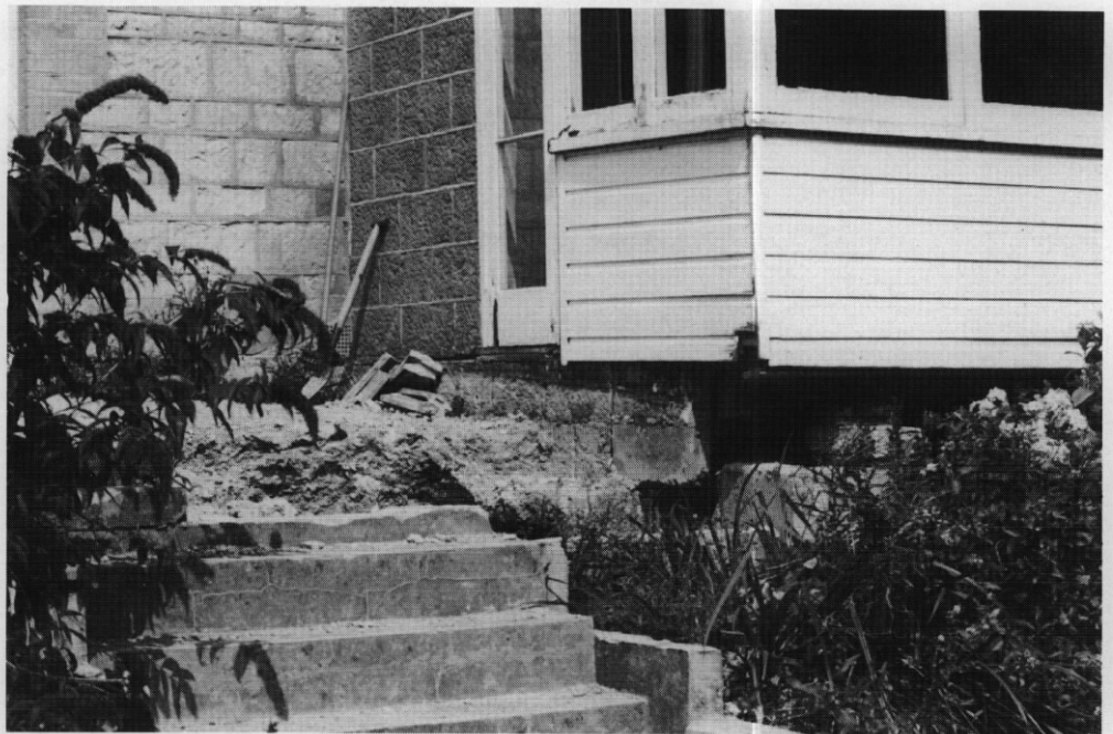
Plate 10. Settlement of foundations at crest of steep slope.
