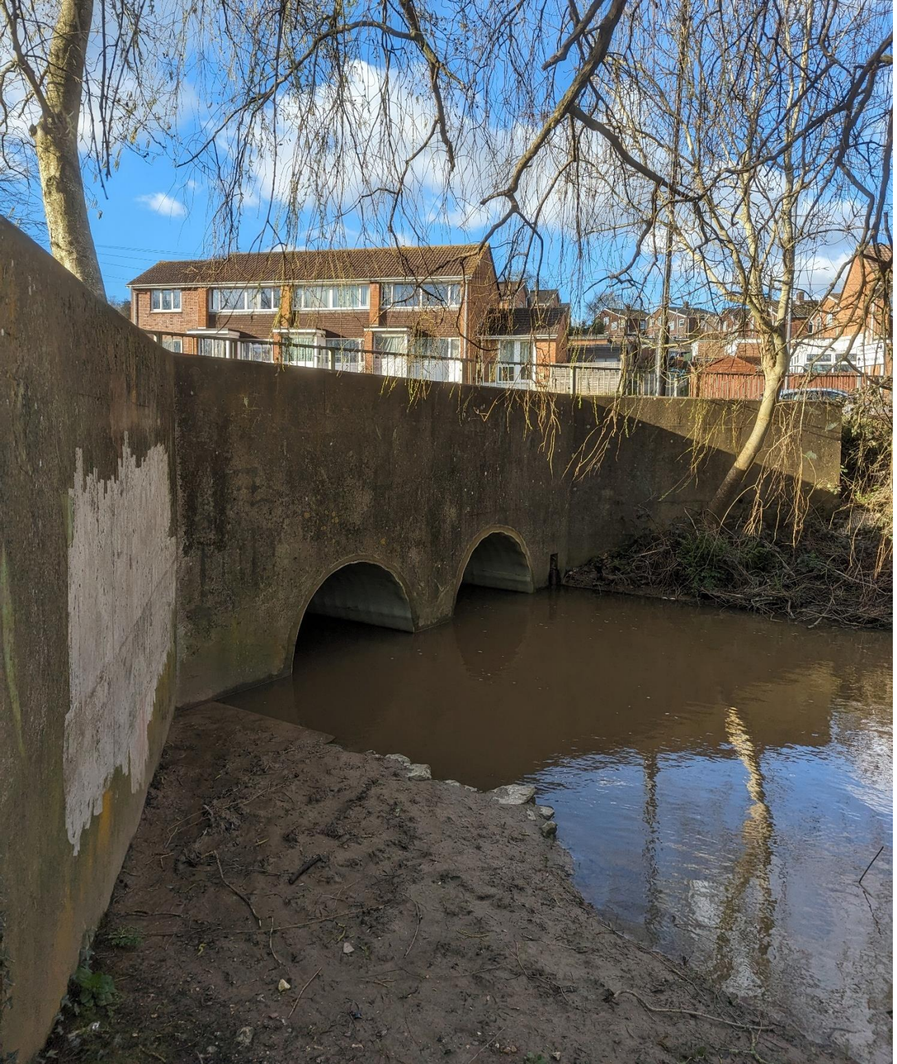
Figure 8-9 Downstream headwall and twin culvert connecting to St James St Duck Pond
