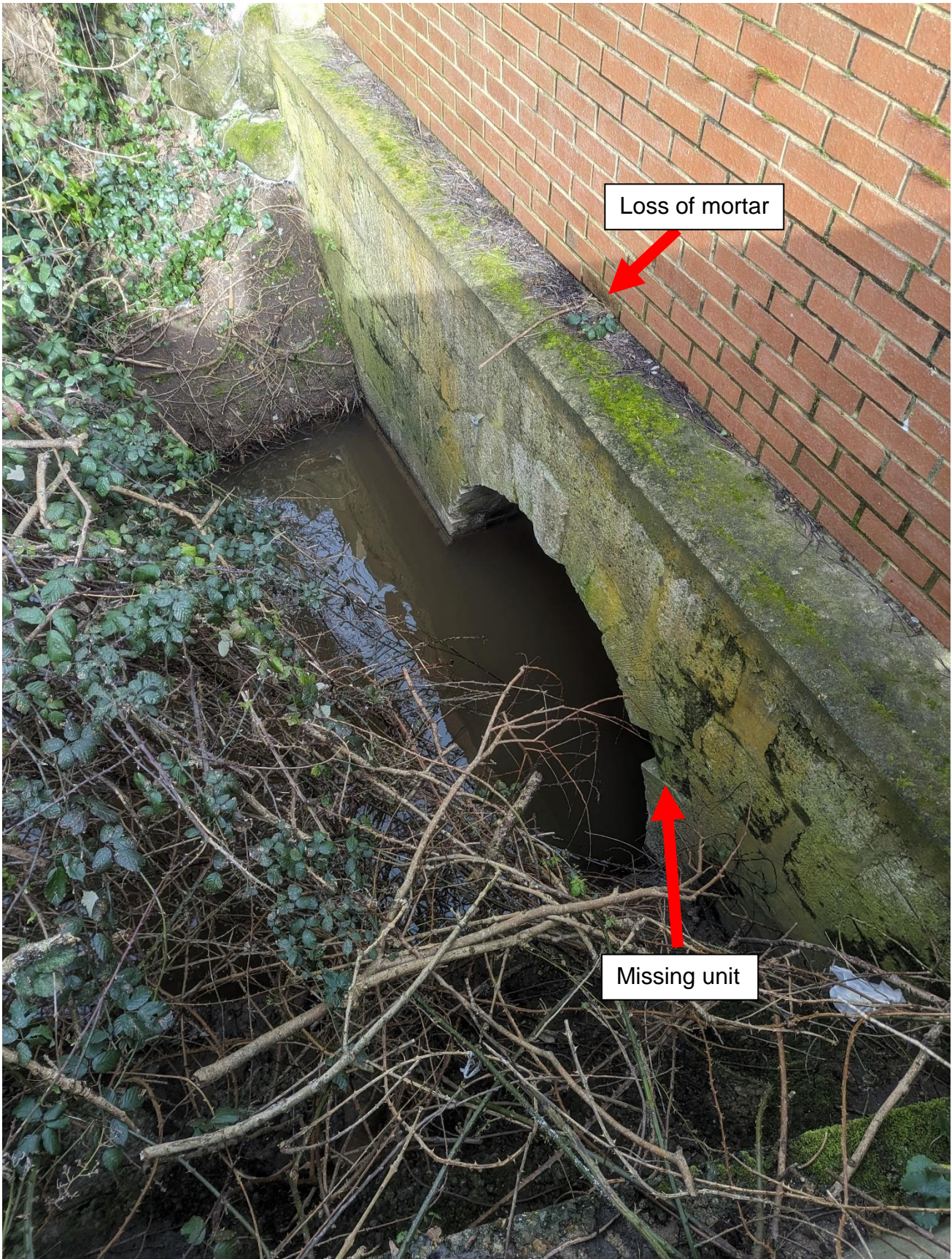
Figure 8-1 Upstream headwall of culvert – picture was taken from the right bank of the asset in front of the back garden of the Ash Lane properties
