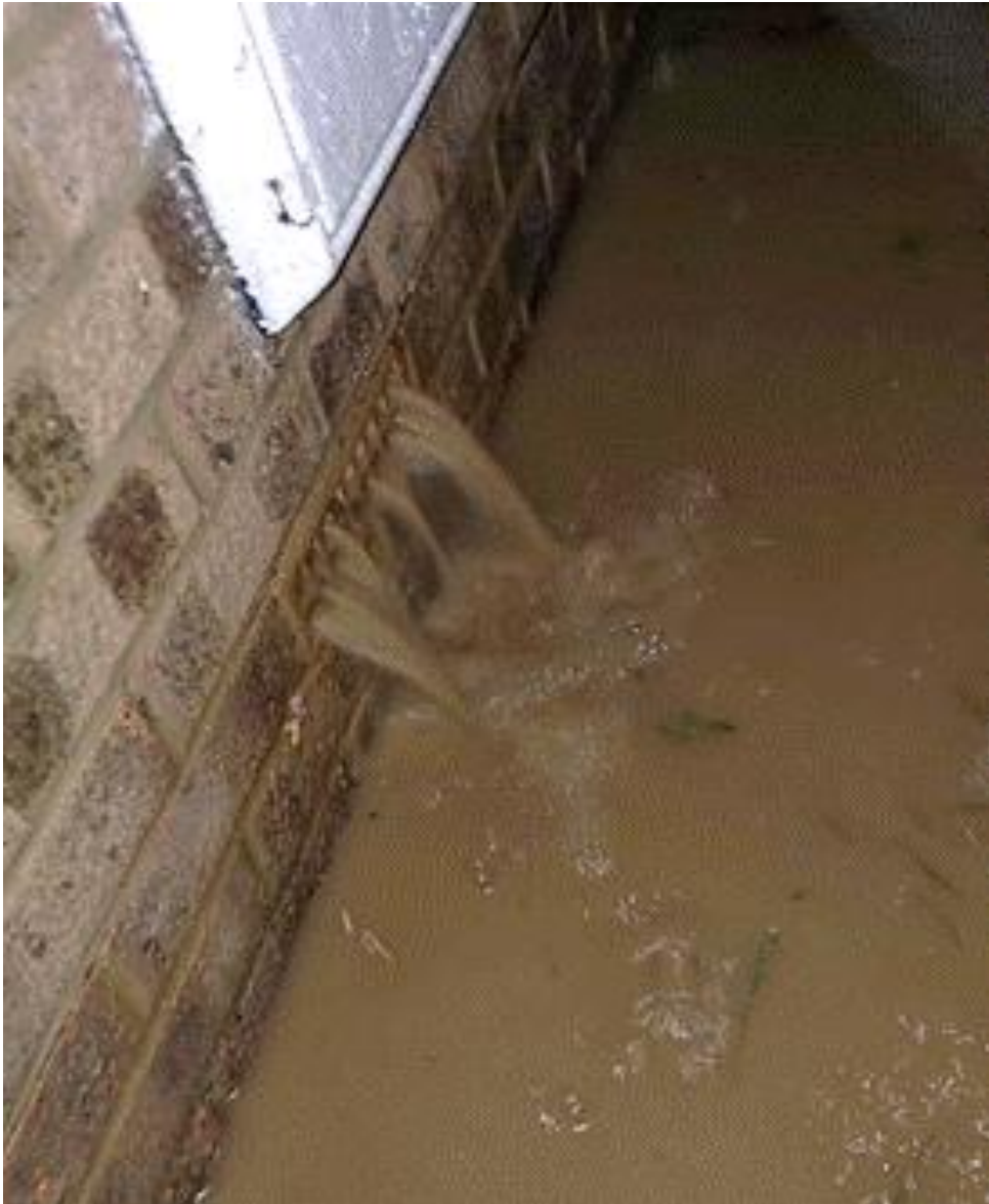
Figure 9-2 Photograph of flooded air bricks, Broadwood Lane
