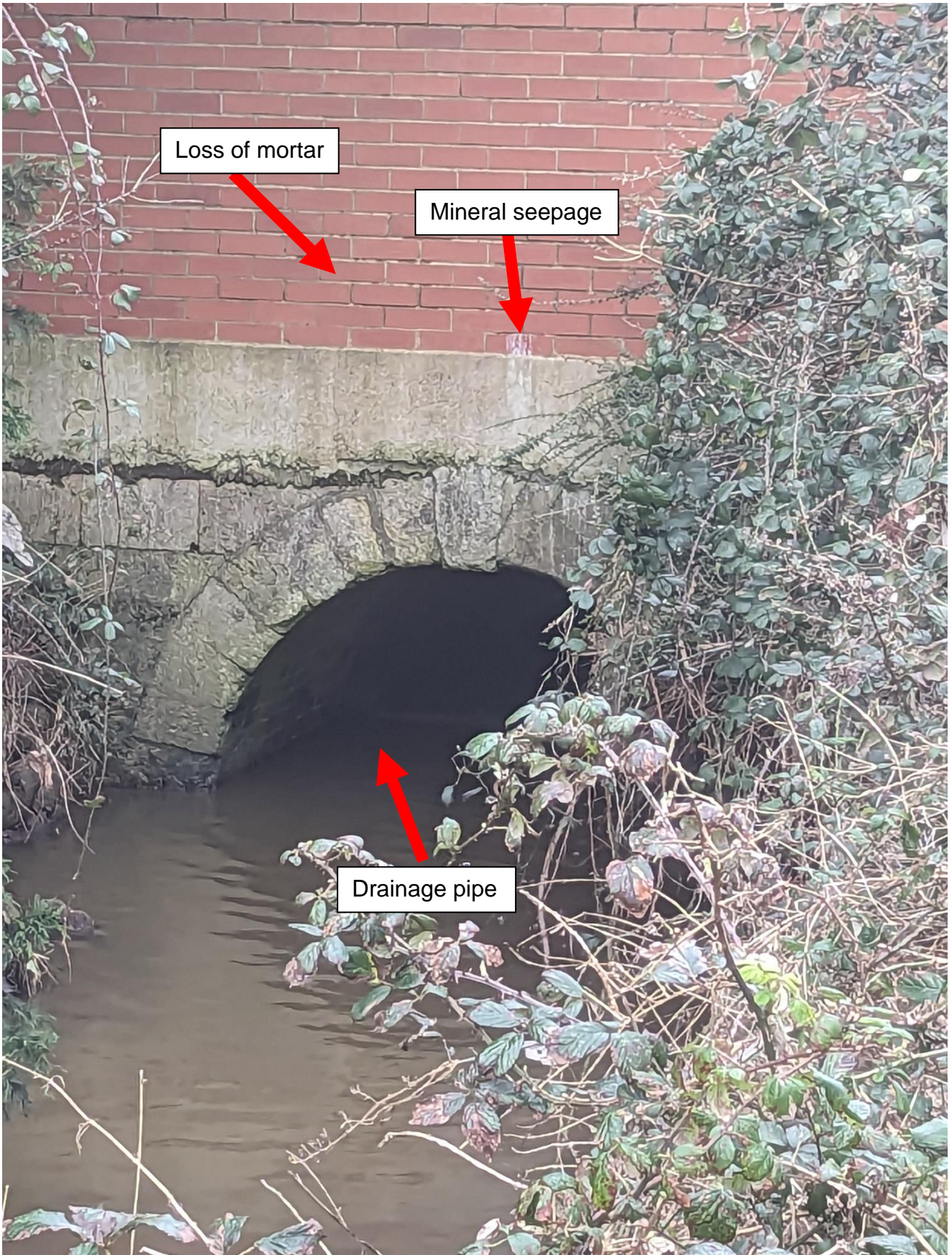
Figure 8-2 Downstream headwall of culvert - picture was taken from the public footpath on left bank
