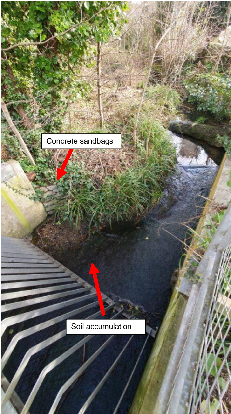
Figure 9-4 Natural high ground and debris screen, looking northeast from the left bank
