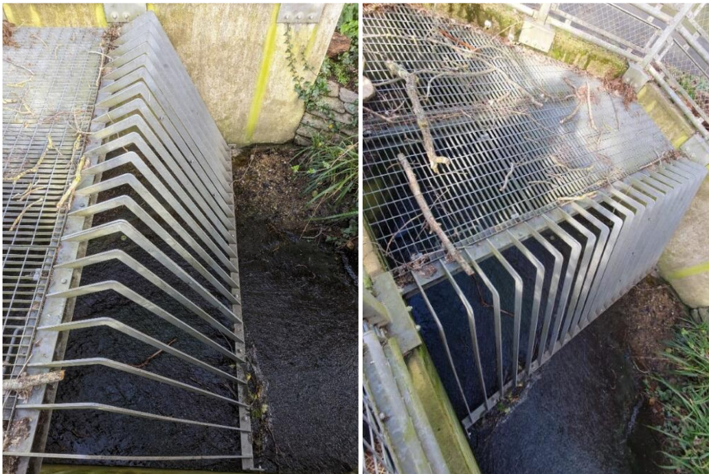
Figure 9-2 Debris screen, looking at asset from the left bank
