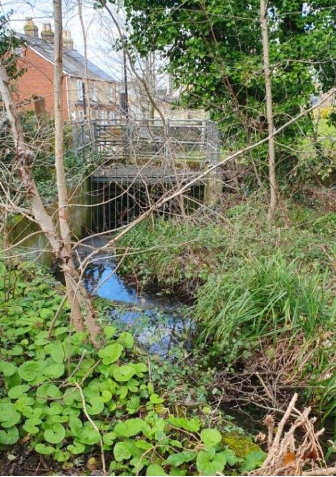
Figure 2-2 Simple culvert with debris screen along main river at Church Path (looking west) during normal conditions.
