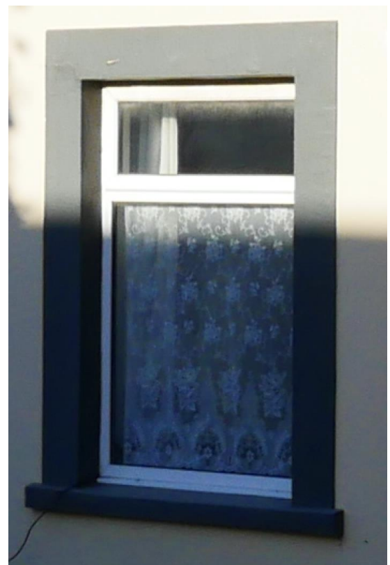
Figure 5 – Inappropriate configuration of replacement window.
