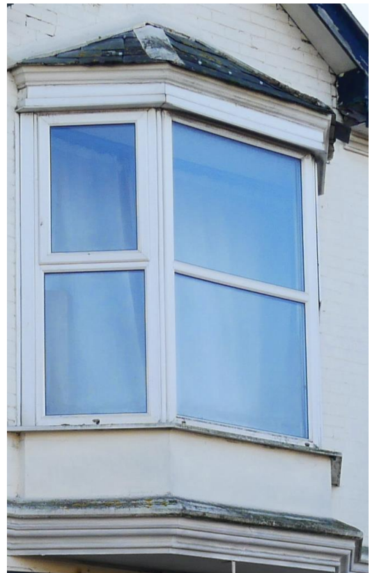
Figure 4 - Poor quality Upvc sash windows to a first floor bay window.
