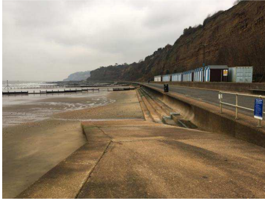
Figure 4-6. Photo (February 2017) showing low beach levels at the central section of the study site. The beach levels are low enough to expose 4 steps of the concrete revetment, which is buried elsewhere in the study site.
