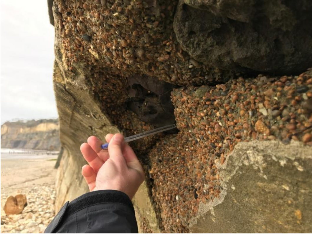
Figure 4-5. Close up photograph of the seawall condition at Shanklin (IW27 005).
