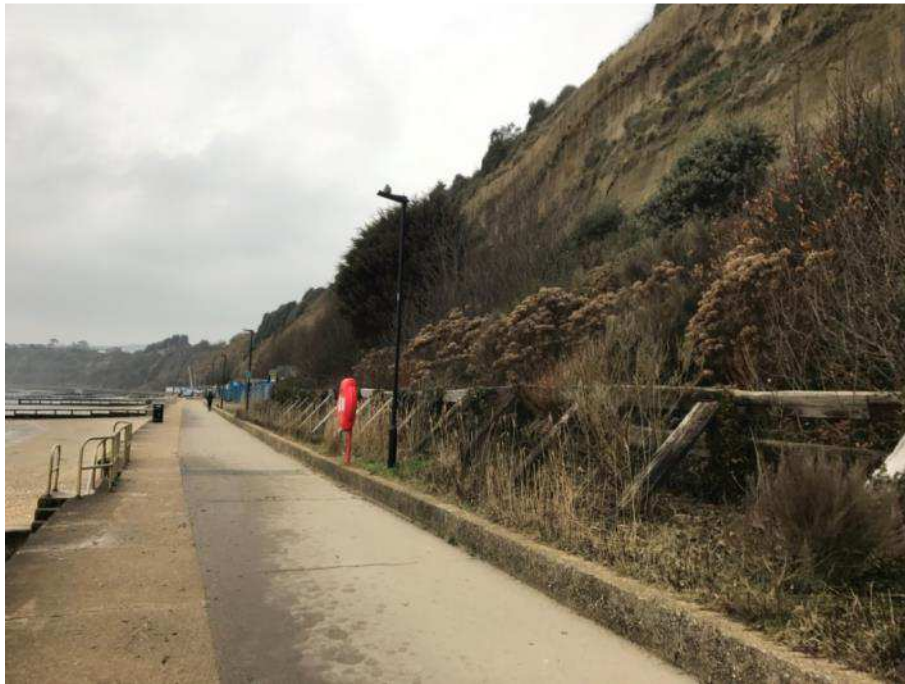
Figure 2-3. Sandstone cliffs and catch fencing between Sandown and Shanklin (February 2017).
