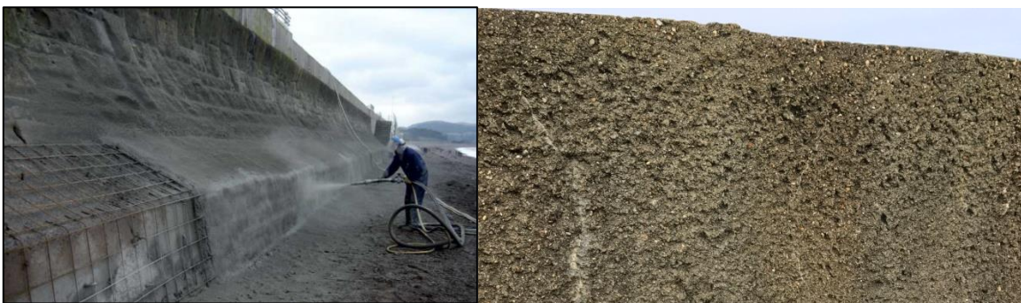
Figure 4-1. Photographs showing examples of concrete spraying of a seawall at Minehead (left) and at Yaverland on the study frontage (right) used to prolong the service life of the asset.
