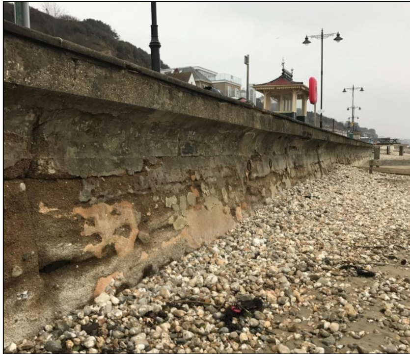
Figure 3-2. IW27 seawall in poor condition (southern end of the esplanade)
