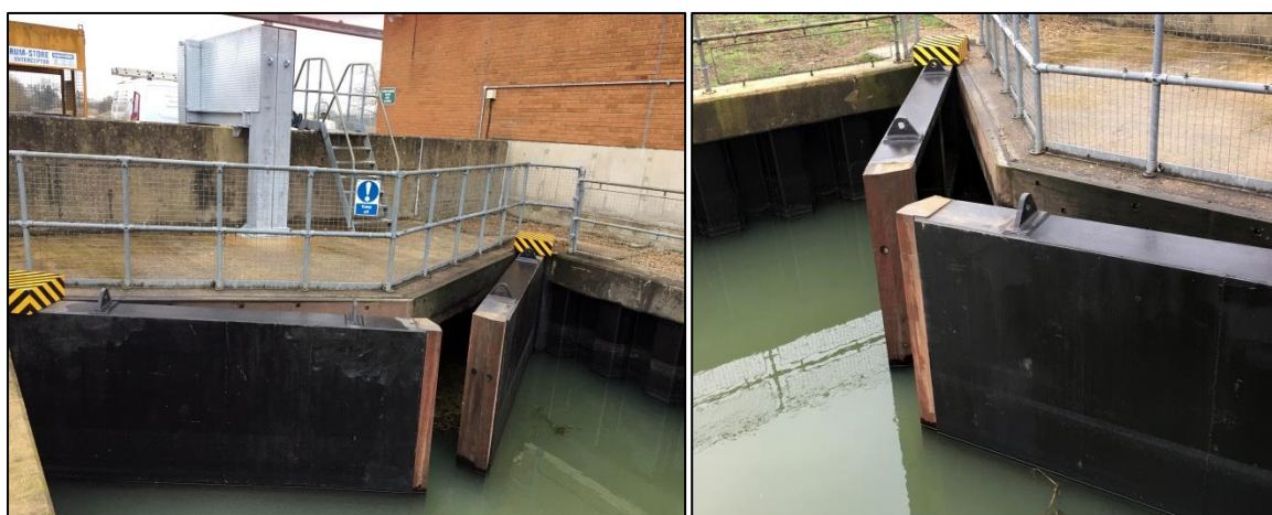
Figure 4-4. Example of flood gates which could be used to mitigate high tidal levels.
