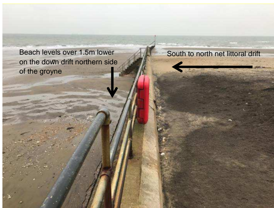
Figure 4-10. Concrete terminal 'Hope' groyne near Shanklin trapping significant volumes of littoral sediment on its southern side (February 2017).
