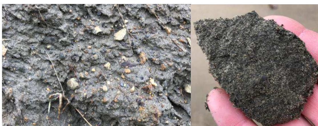
Figure 4-4. Photographs showing the composition of the cliffs south of Shanklin Chine (site visit March 2017)
