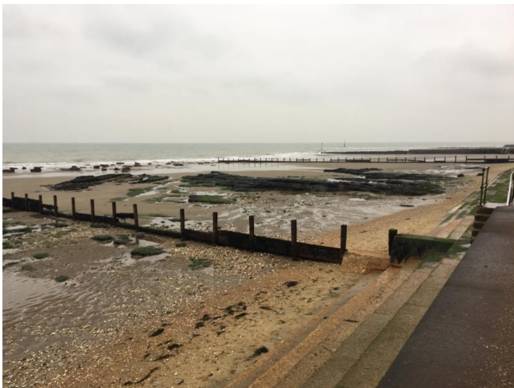
Figure 4-2. Photograph showing the groynes and exposure of wave cut platform (at Lake)
