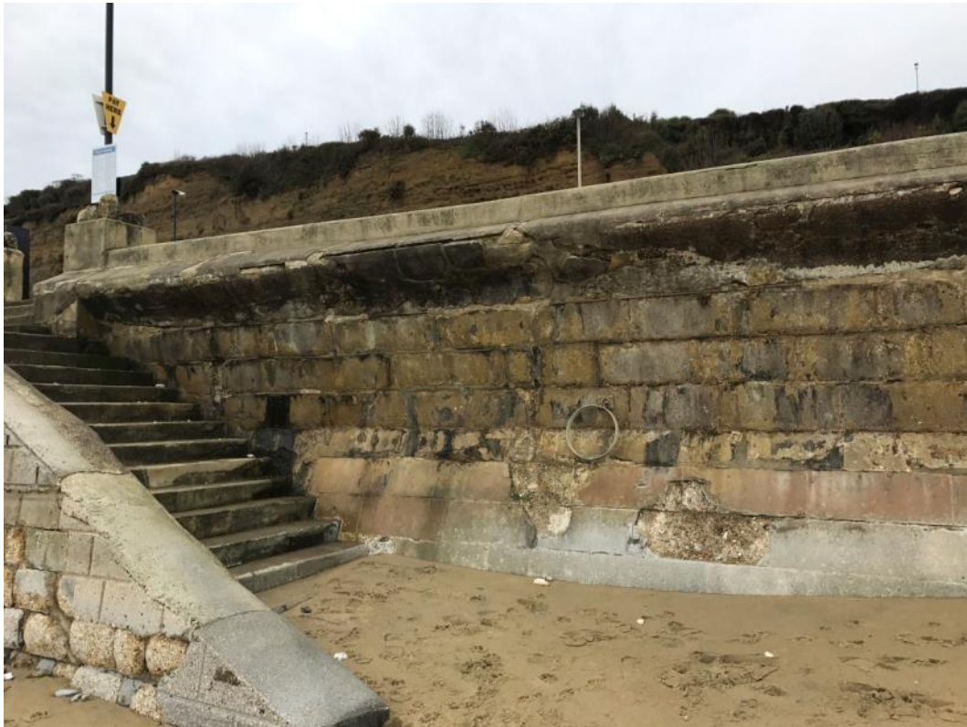
Figure 4-3. Photograph showing the seawall at North Shanklin (in-front of the 'crazy golf' area) - IW27 002.
