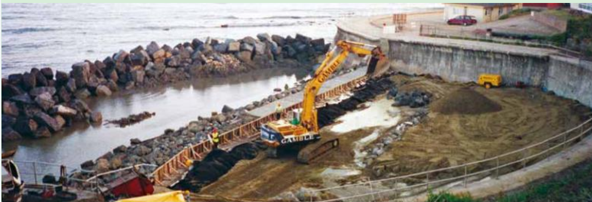
Constructing the new coastal defences seaward of the existing wall in order to provide support for the slope behind.
