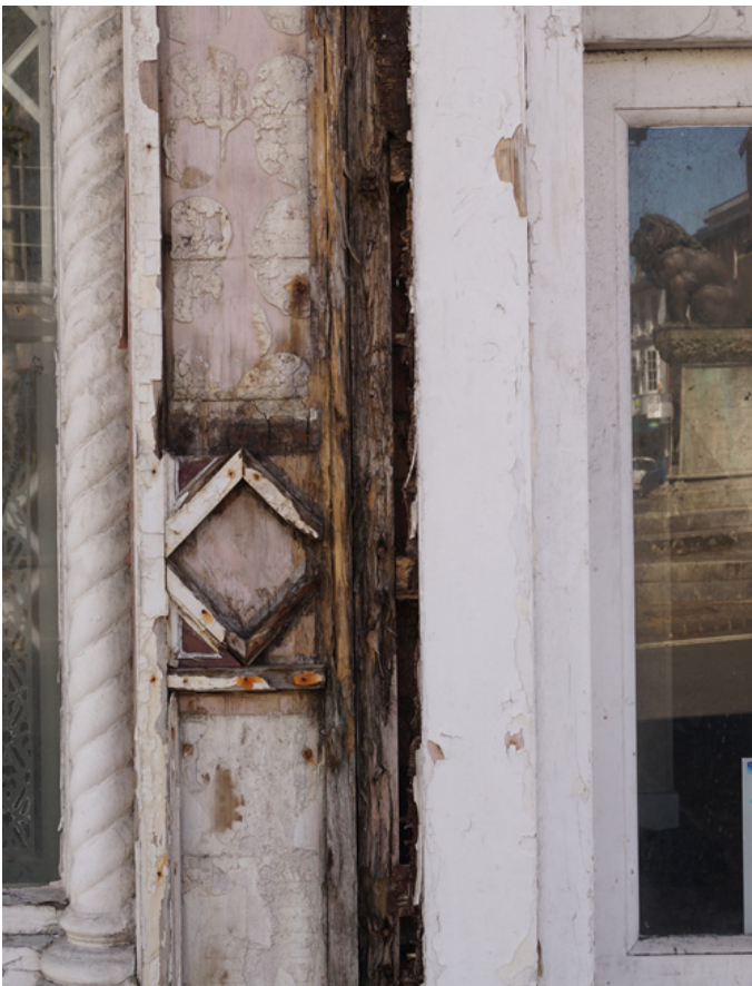
The effects of poor maintenance can clearly be seen on this shopfront joinery
