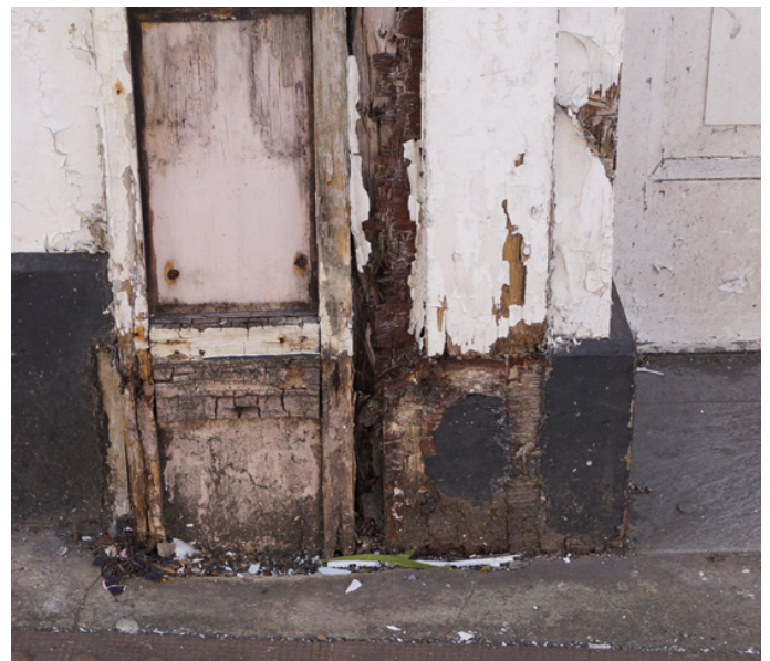
Timber stallriser suffering from bad damp
