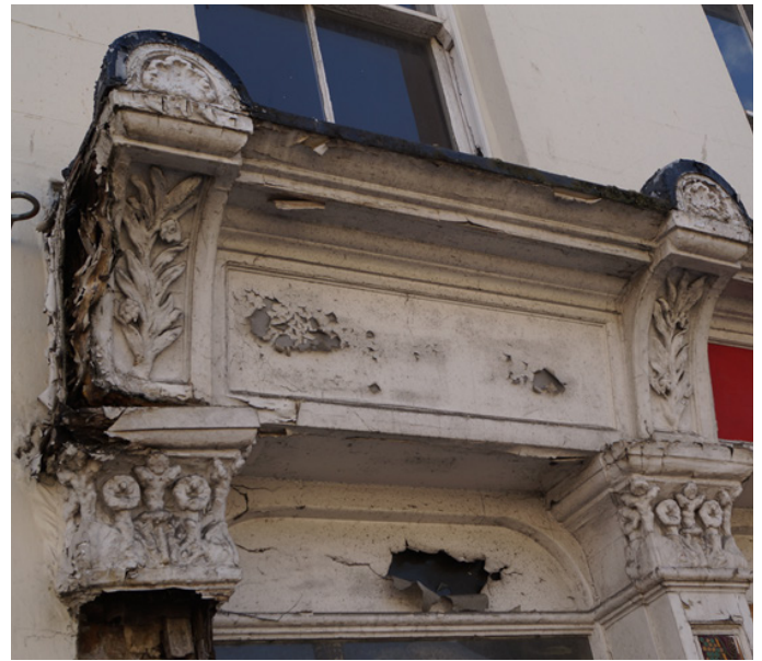
A poorly maintained traditional shopfront in Newport
