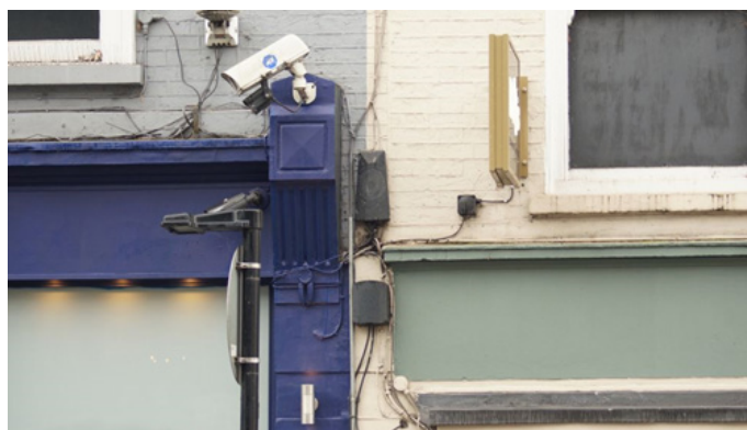
A poor example of electrical wiring and electronic devices cluttering a shopfront, London.
