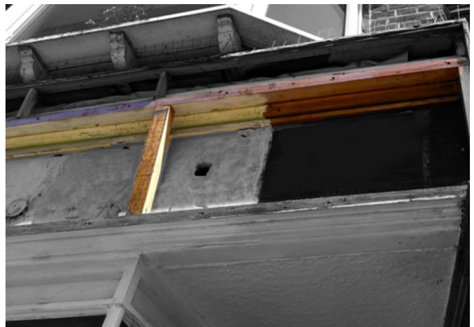
An example of an additional horizontal, timber batten supported by vertical post and used to achieve an angled fascia.
