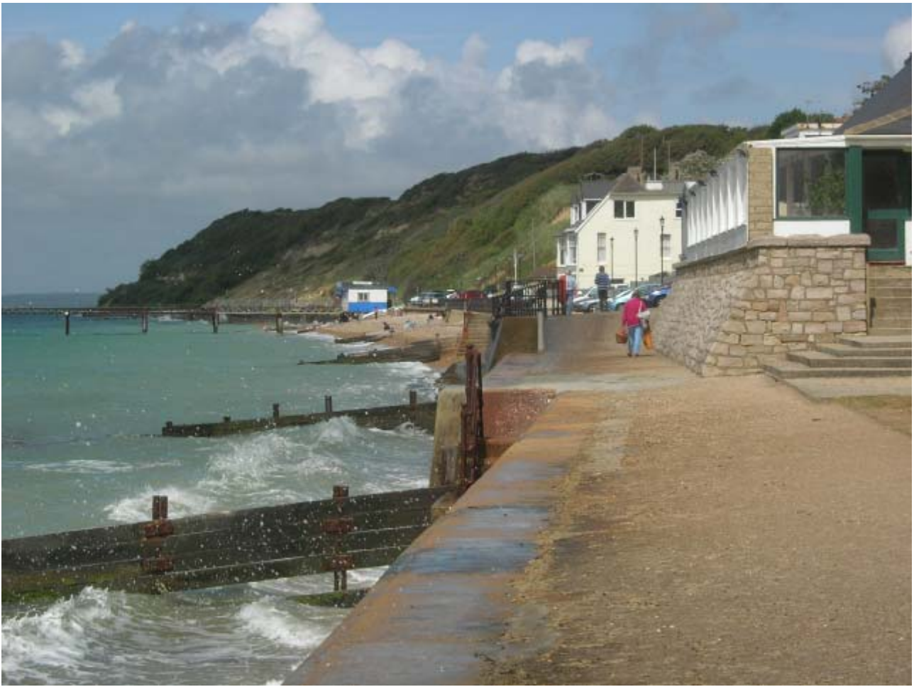
Plate 24: Totland Bay, where cliff reactivations have slumped over the seawalls. July 2009
