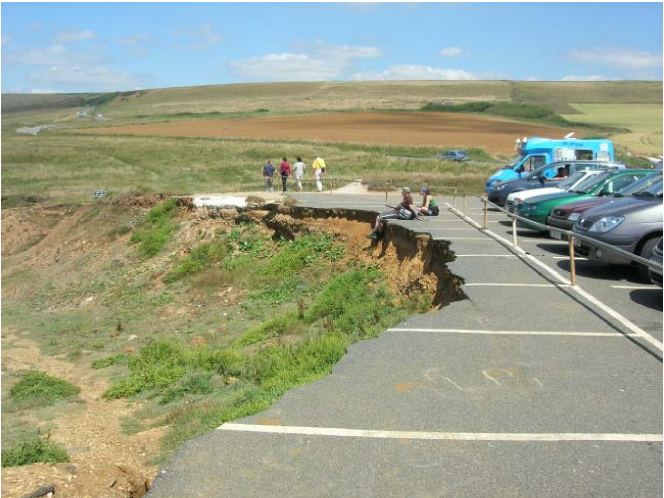
Plate 19: Erosion of the car park behind Compton Bay, July 2006.
