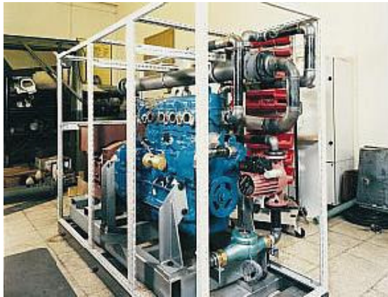
Figure 7 Package Gas Engine CHP Unit
