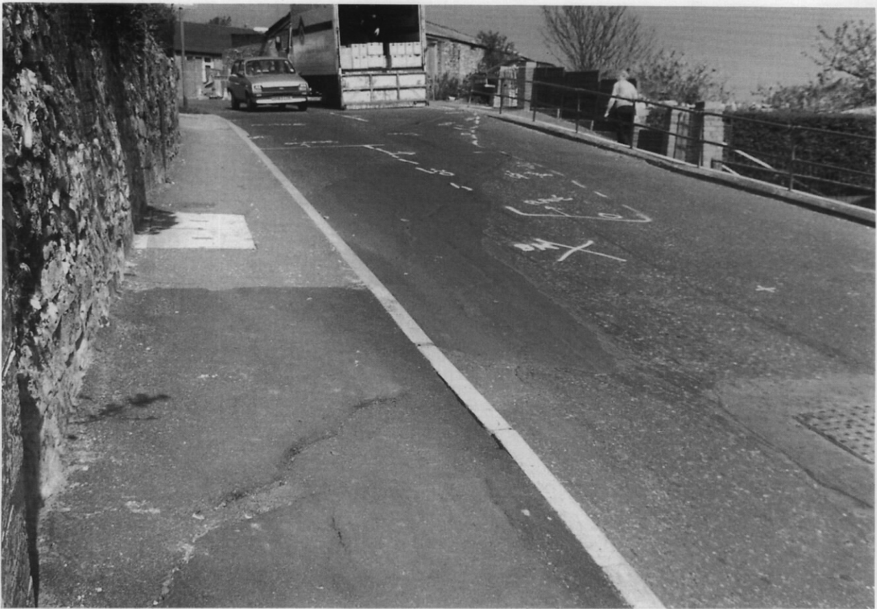
Plate 2: Within the "graben", roads and hardstandings require regular repair
