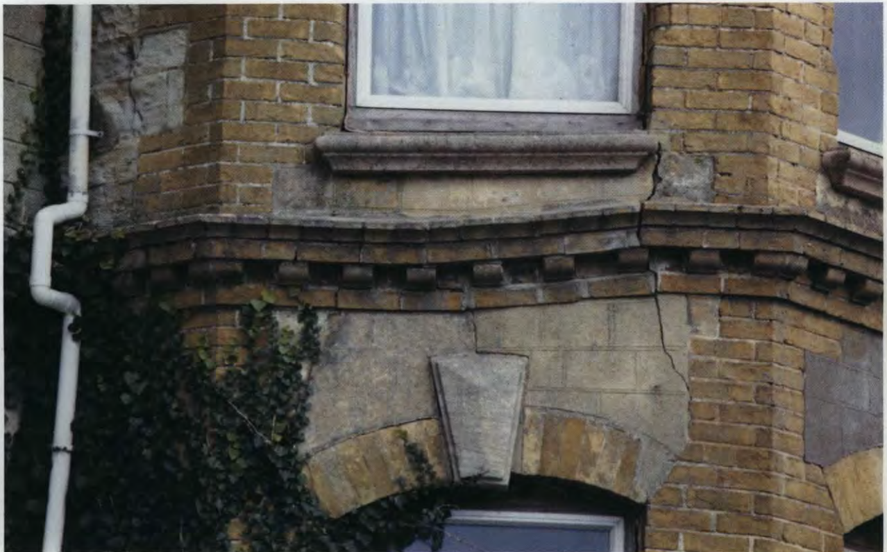
Plate 6: Structural damage has caused misalignment of the string course and also displacement of the arch and keystone
