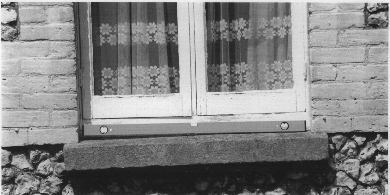
Plate 15: Differential ground movement has distorted the frame and tilted the sill
