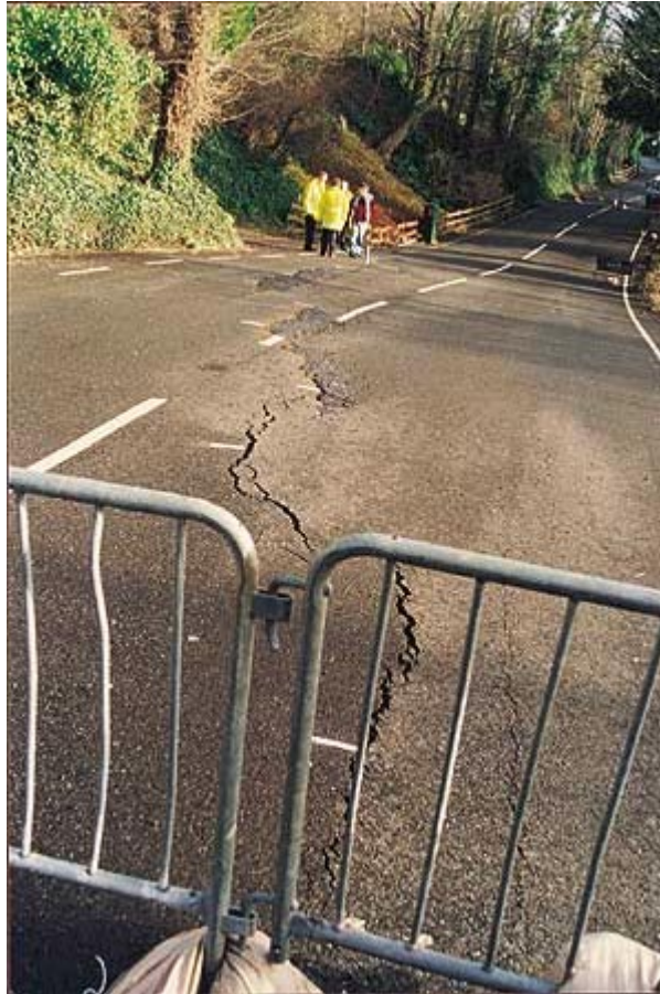
Plate G6a Damage to the main road A3055 at Woodlands
