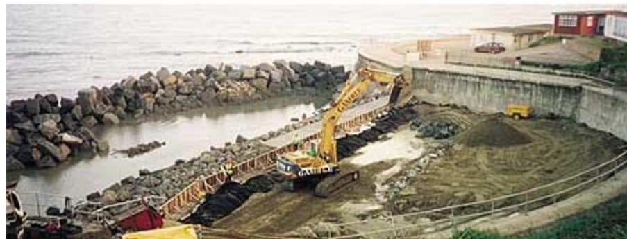
Plate 5b Coast protection and slope stabilization works in progress, 1999 (Courtesy D.Bowie Photography)
