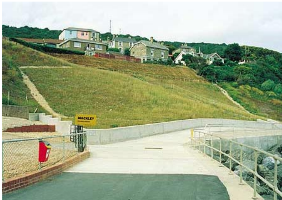
Plat G5f The completed coast protection and slope stabilization scheme after a successful growth of grass, August 2000
