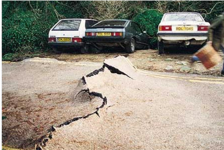
Plate G8e Road damage at Blackgang
