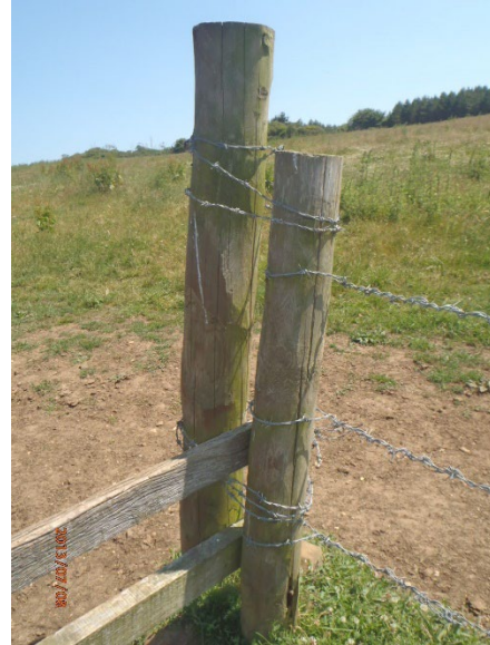
Poor example – barbed wire must not be attached to any part of a stile or gate, including supporting posts – dangerous to users X
