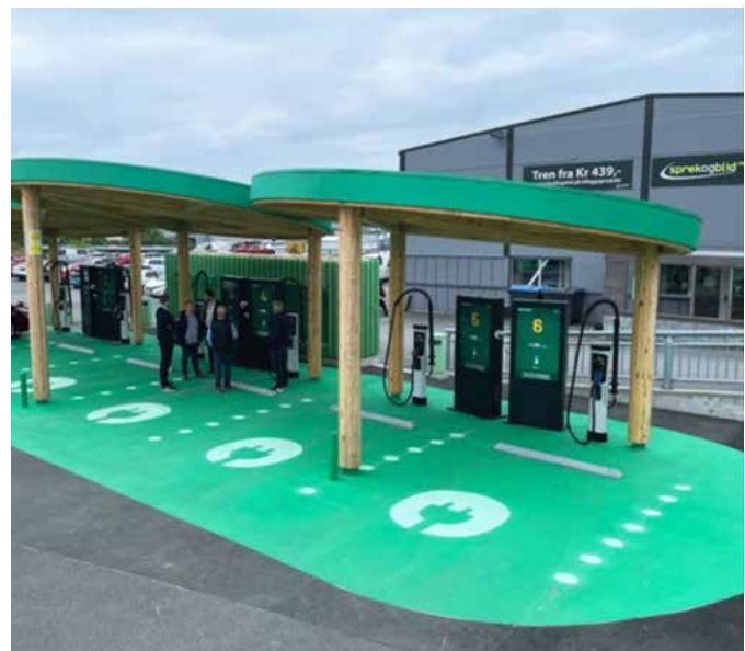
Figure 15: Greenstation charging hub (Photo courtesy of Greenstation)
