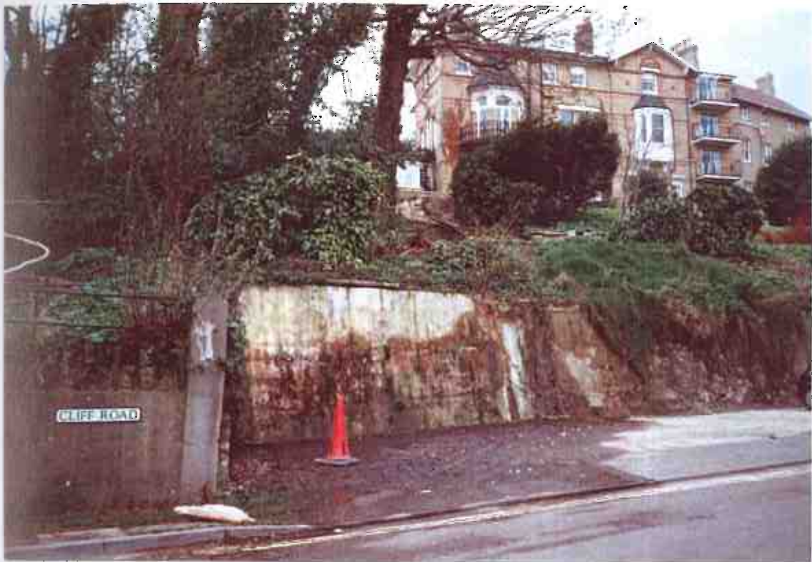
Groundwater seepage and general decay of retaining wall (serious damage)
