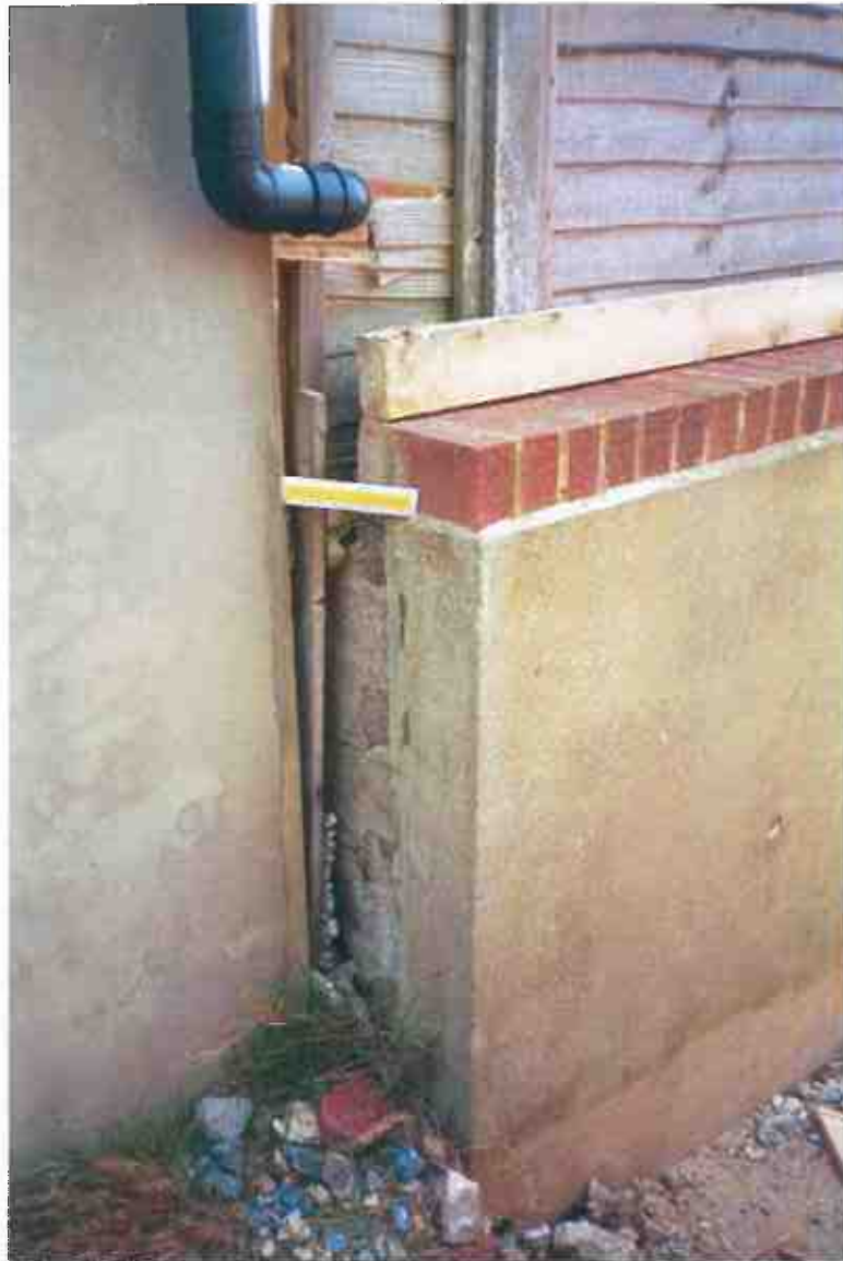
Separation and outward displacement of podium (serious damage)
