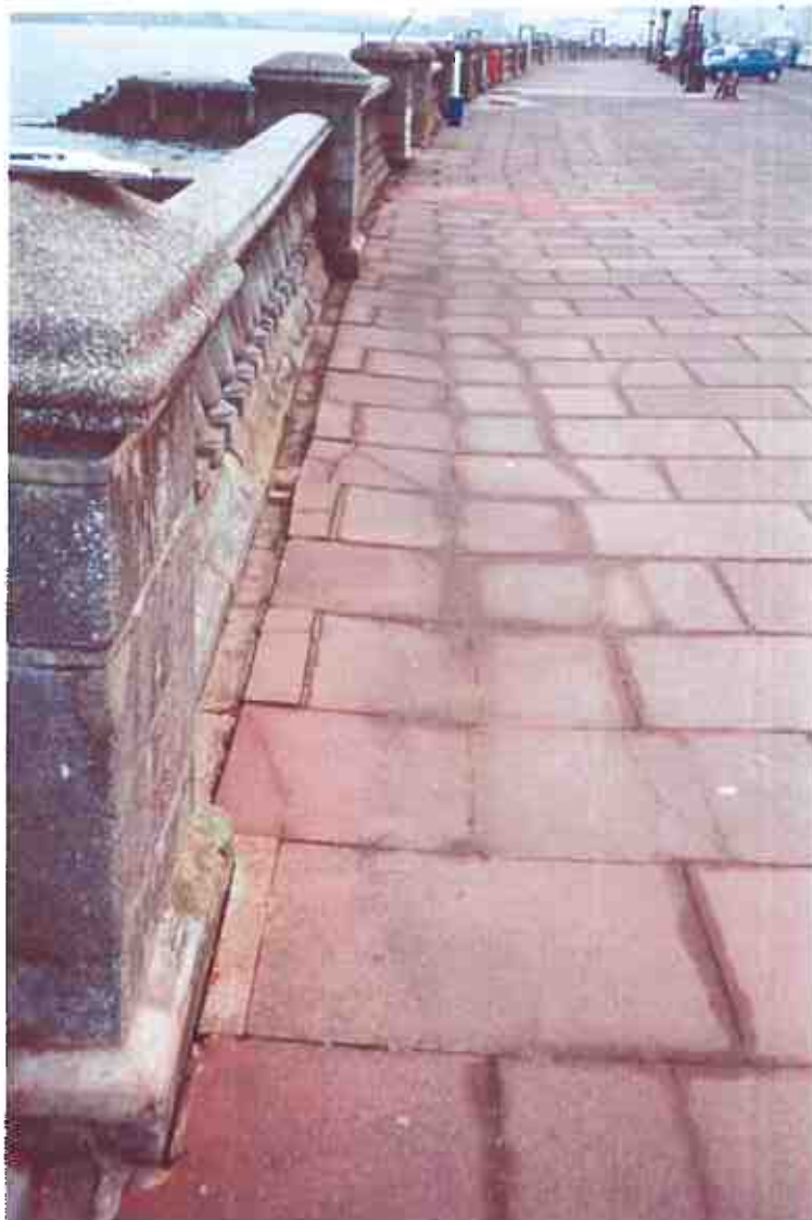
Subsidence and crack damage to the Parade, Cowes (moderate damage)
