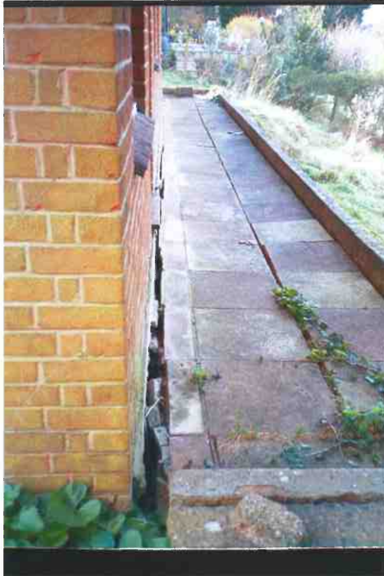
Separation of podium from main structure (serious damage)
