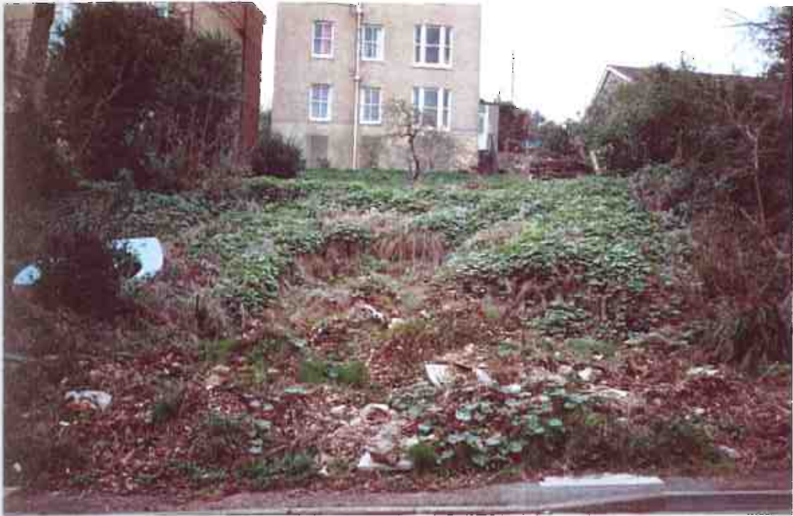
Small failure of garden slope (severe damage)
