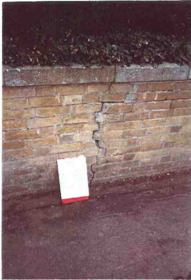
Crack damage to low boundary wall (moderate damage)
