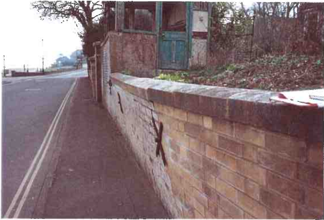
Forward tilt and heave of walls and outbuilding (serious damage)
