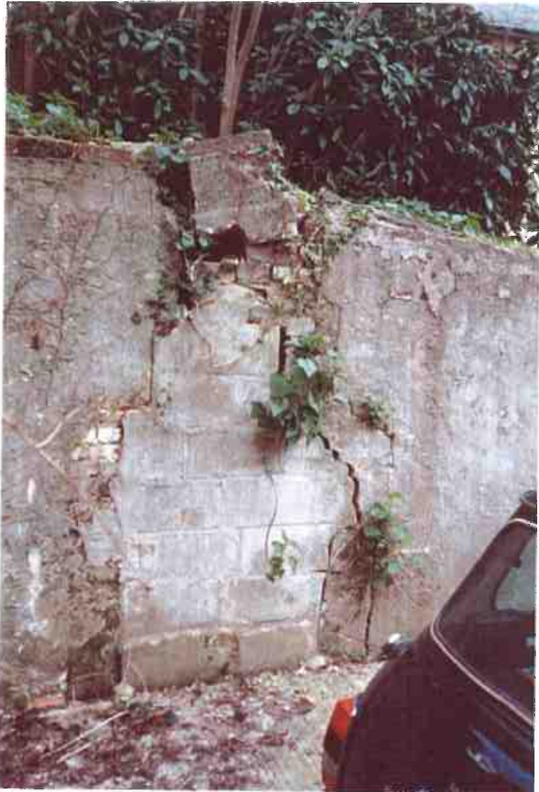
Crack damage and dislodgement of masonry blocks (serious damage)
