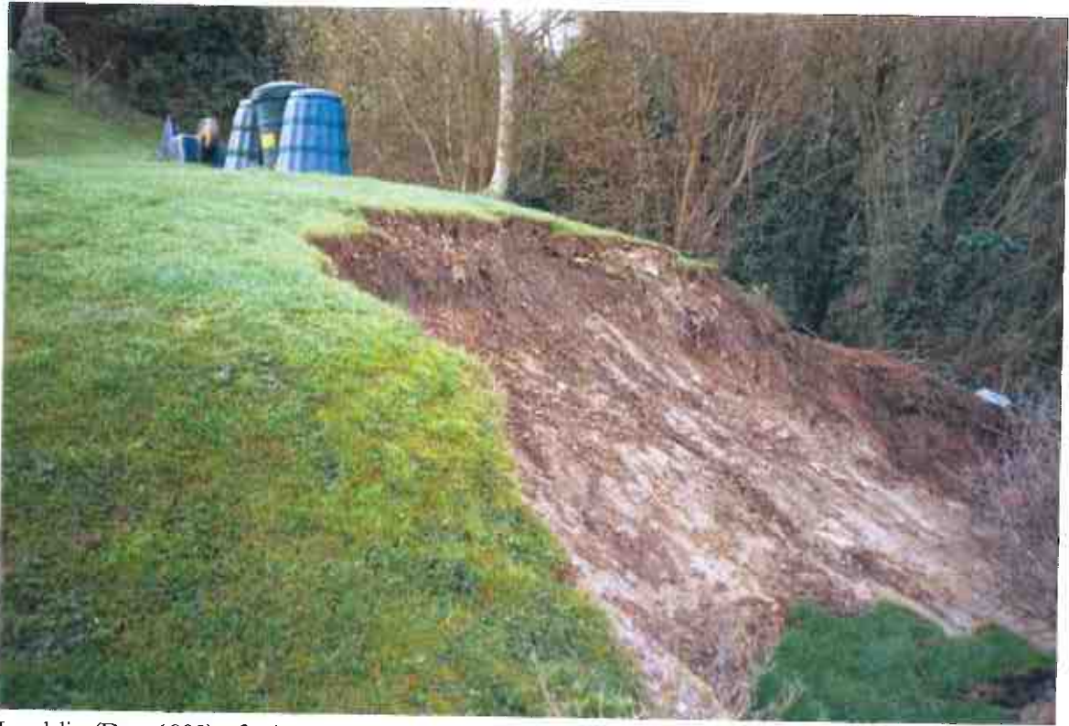
Landslip (Dec. 1999) of private garden at crest of coastal slope (severe damage)
