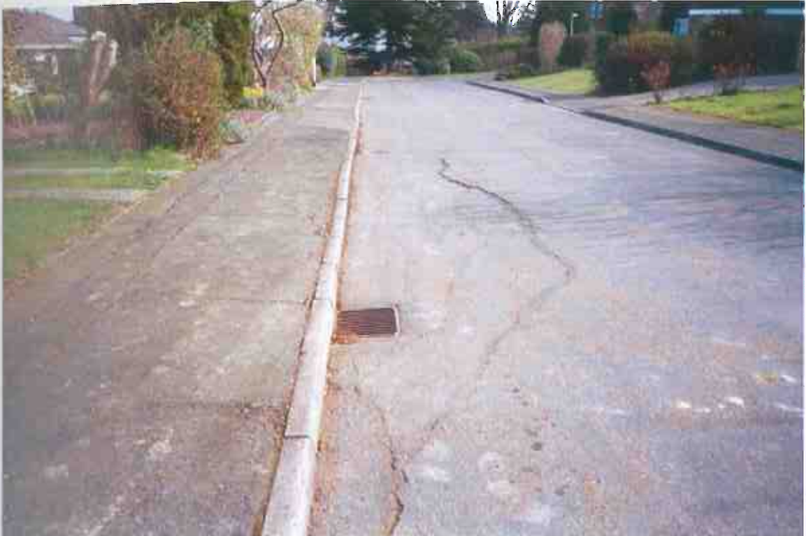
Subsidence and crack damage of road pavement (moderate damage)
