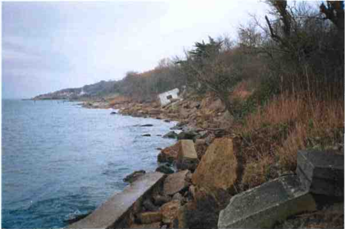
Plate 5 Collapsed Private Coastal Defences at Gurnard Cliff
