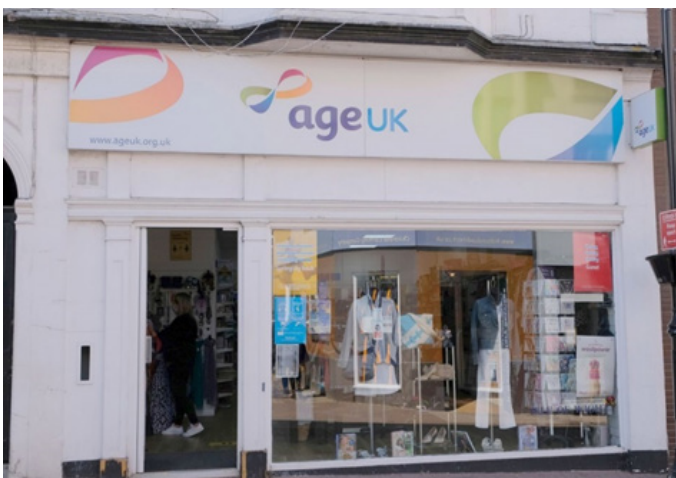
A poor example of a modern fascia mounted on, and obscuring architectural detail of heritage value.
