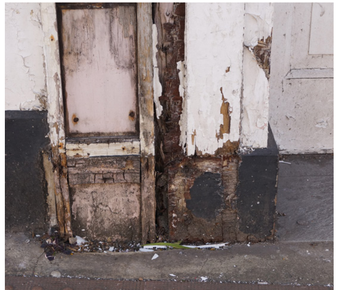
Timber stallriser suffering from bad damp
