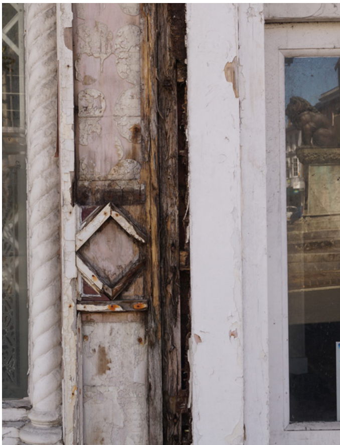
The effects of poor maintenance can clearly be seen on this shopfront joinery
