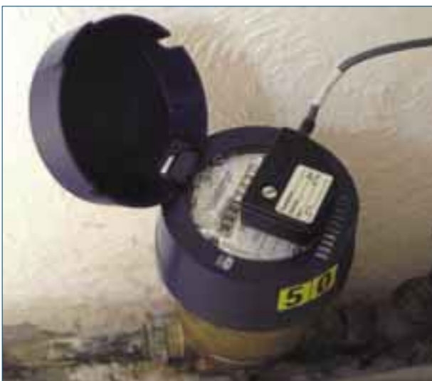
Domestic Water Meter
